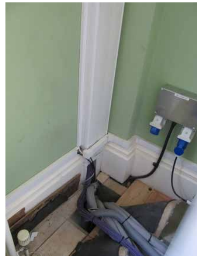
Figure 7 - Large amounts of services are currently run within the floor voids to enable the building to be used as offices
