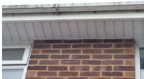
6. Soffits boxes around the eaves of the house sealed tightly to the brickwork walls and window frames.
