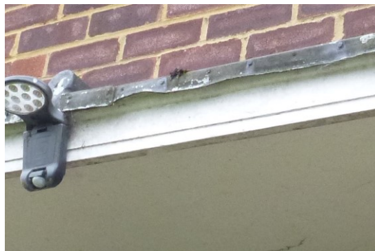
8. Narrow gap behind lead flashing on the porch to the front of the house.
