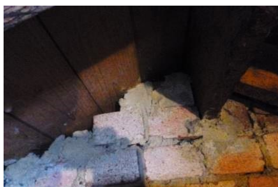
12. Gaps visible around the internal dividing wall.
