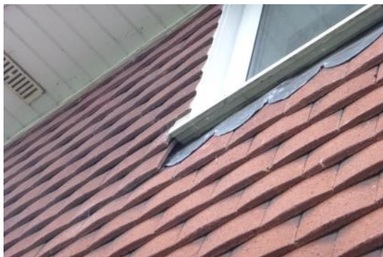
7. Gaps behind hanging tiles around window to the front of the house.
