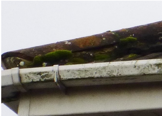
5. Mortar missing from a hip tile to the rear of the house.
