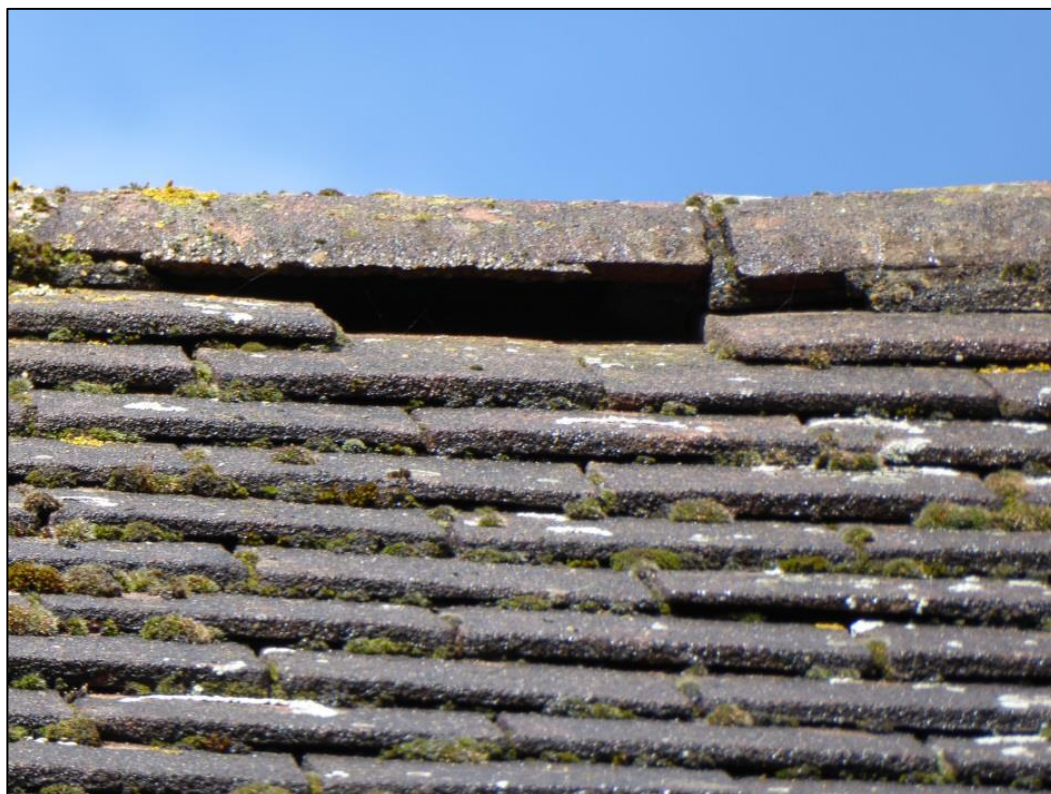
Figure 7. 26 Woods Road, Gasp in ridge. 15.09.15.
