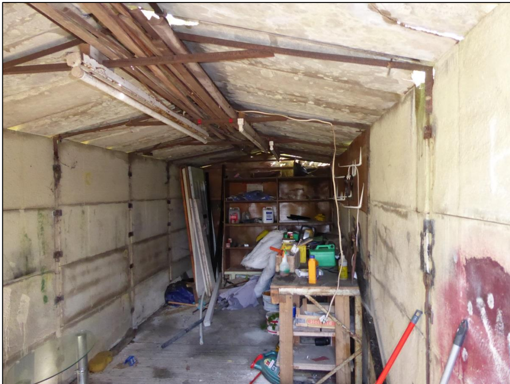
Figure 10. 26 Woods Road, internal view with gaps in garage roof, 15.09.15.
