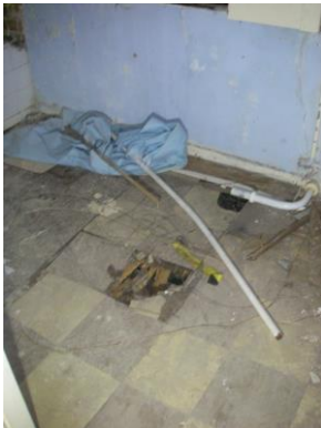
Photograph 15: Rotten floor to bathroom adjacent G6
