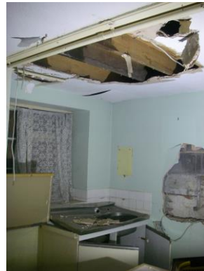
Photograph 16: Exposed ceiling/floor joists and wall break out in G6
