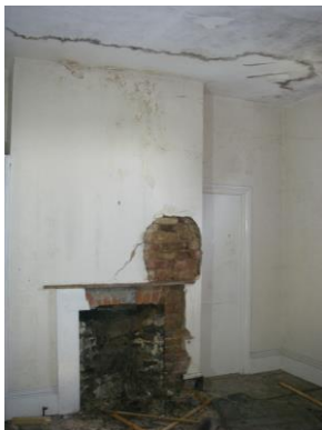
Photograph 23: Water damage and damp, crumbly brickwork to chimney breast in F4
