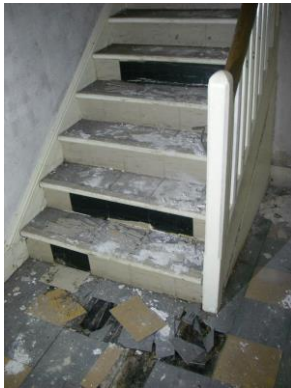
Photograph 25: Rotten/collapsed floor at base of stairs in Stair 2
