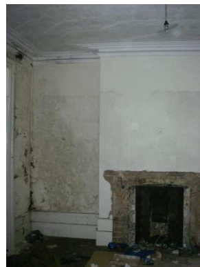
Photograph 6: Damp in corner of room G2
