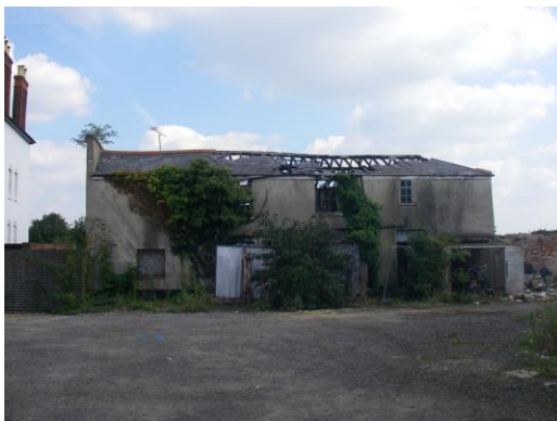
Photograph 40: Dilapidated fire damaged building
