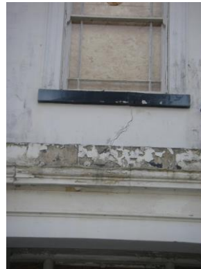
Photograph 31: Crack over portico up to window cill above
