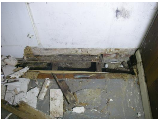
Photograph 17: Removed floor boards in corner of G7
