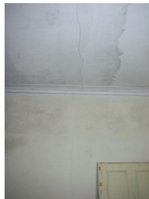
Photograph 18: Crack in ceiling and wall in F1
