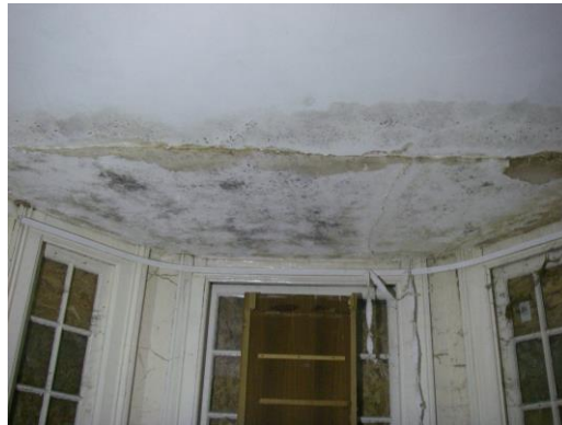
Photograph 13: Water damage to ceiling in bay window in G5
