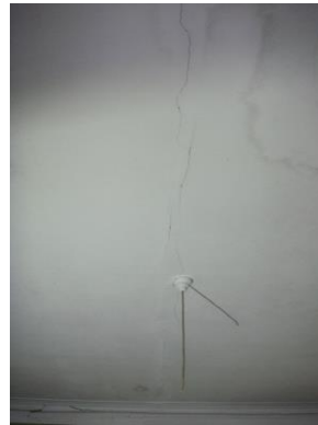
Photograph 20: Crack in ceiling in F2
