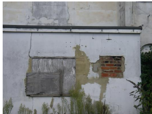
Photograph 35: Bricked up window and cracks in walls single storey addition to rear.
