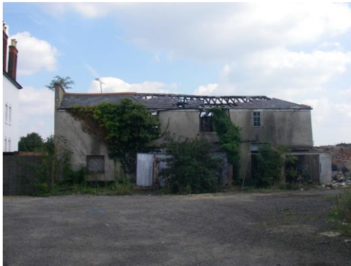
Photograph 2: Dilapidated and fire-damaged separate building
