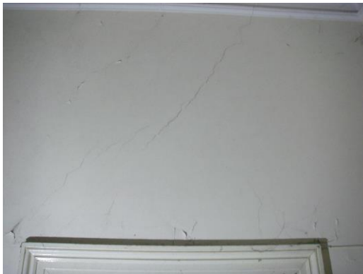
Photograph 9: Cracking over door to G1 seen from Corridor 1
