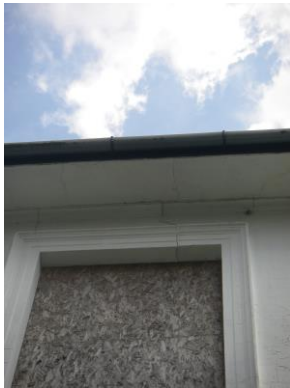
Photograph 38: Cracks above lintels
