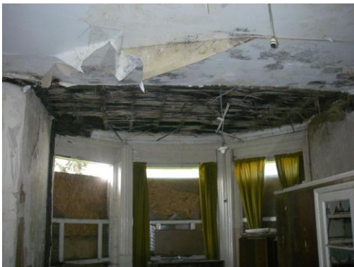
Photograph 4: Collapsed ceiling above bay window in G1
