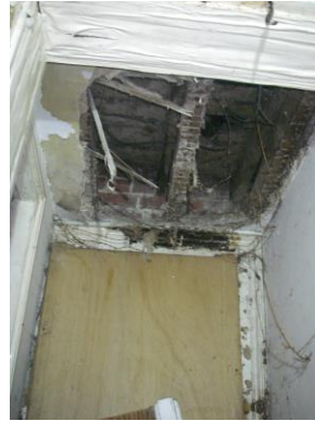
Photograph 8: Collapsed ceiling to WC to rear of Corridor 1
