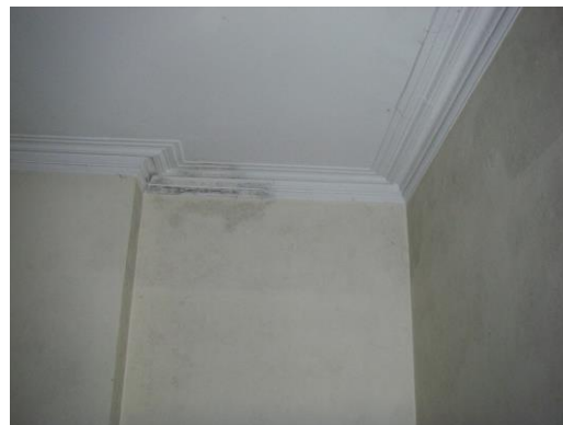
Photograph 10: Localised damp staining in G3
