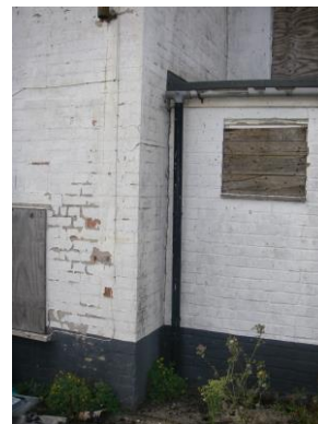
Photograph 33: Crack to entrance porch
