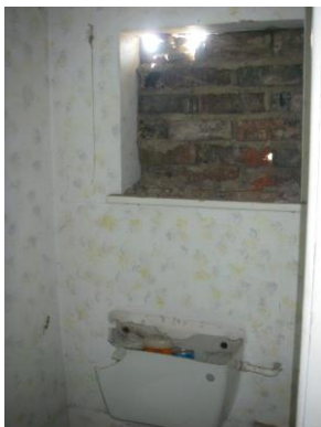
Photograph 5: Bricked up window to WC in rear addition to G2
