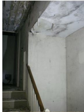
Photograph 26: Ceiling damage in Stair 2
