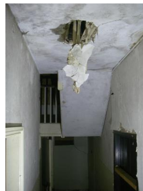
Photograph 12: Ceiling falling in in Corridor 2
