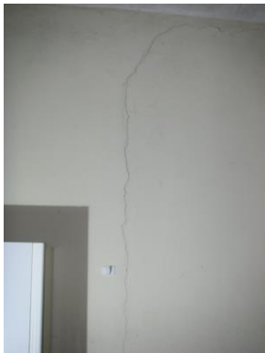
Photograph 21: Crack through wall in Kitchen to F1
