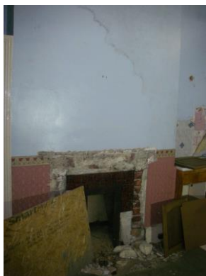
Photograph 11: Water staining to chimney breast in G4
