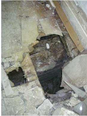
Photograph 7: Collapsed floor adjacent WC to rear of Corridor 1
