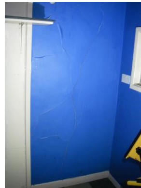
Photograph 28: Crack in wall of F6 adjoining to chimney breast in F4
