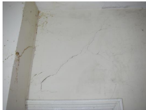
Photograph 24: Cracking in wall over door adjoining to F6, adjacent chimney breast in F4
