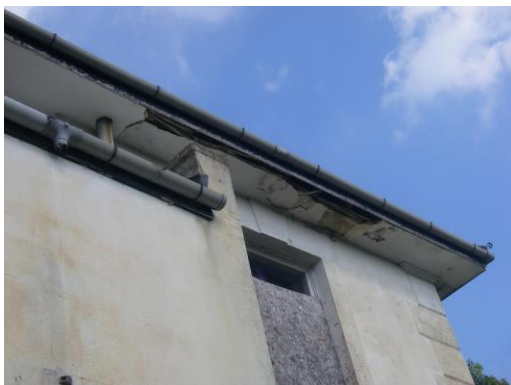
Photograph 36: Rotten eaves soffit on south elevation
