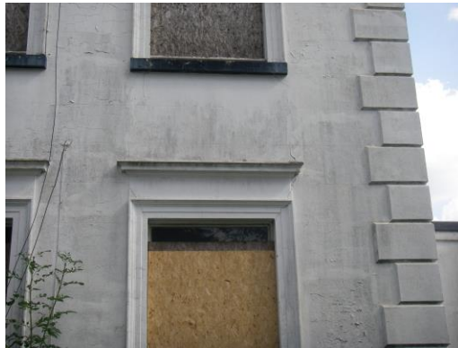
Photograph 37: Crack from lintel to window cill on west elevation
