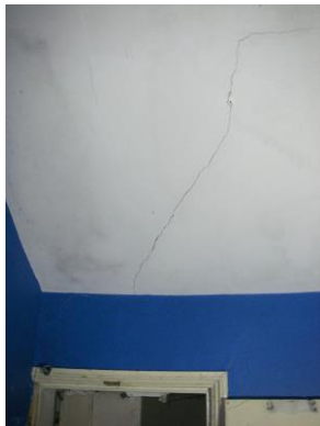
Photograph 27: Crack in ceiling of F6
