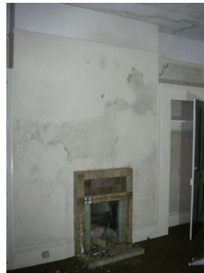
Photograph 22: Staining and mould to chimney breast in F3
