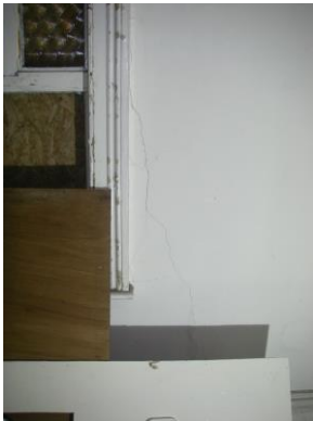
Photograph 19: Crack adjacent window in F1
