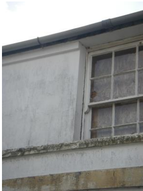
Photograph 32: Cracking around window frames
