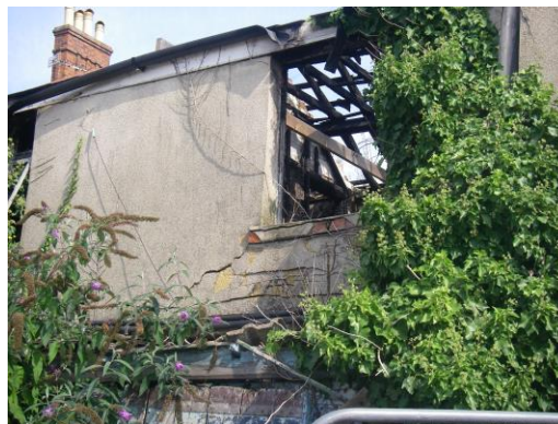
Photograph 39: Damage to dilapidated building
