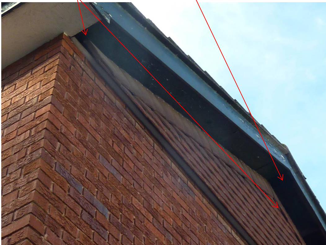
Gaps around hanging tiles and missing section of eaves (front of building – north aspect)
