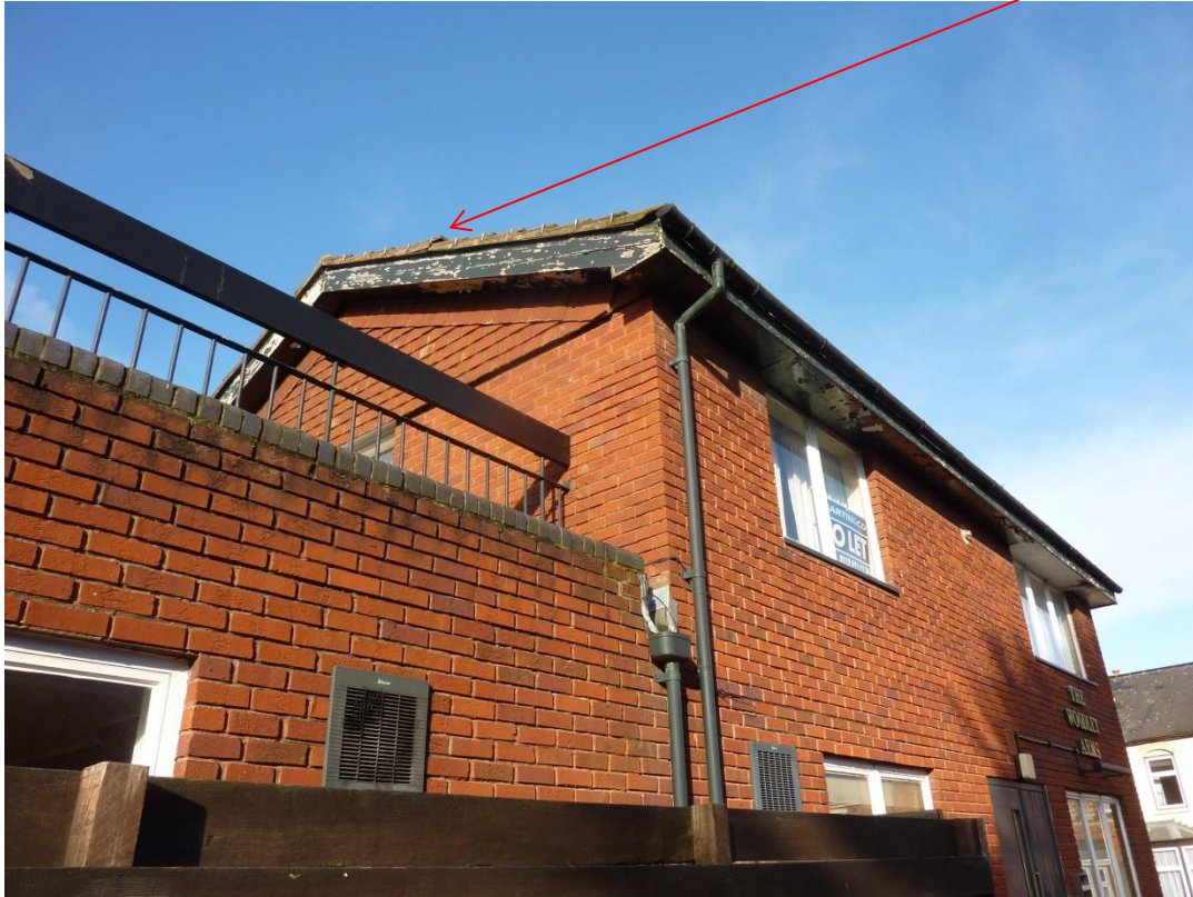
South-east view showing hanging tiles and gap under roof tiles
