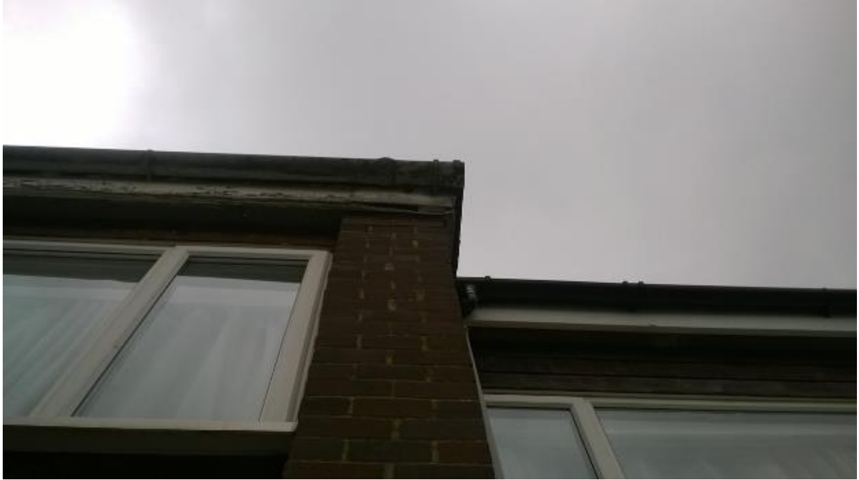
Figure 15: damaged soffit board on B3.
