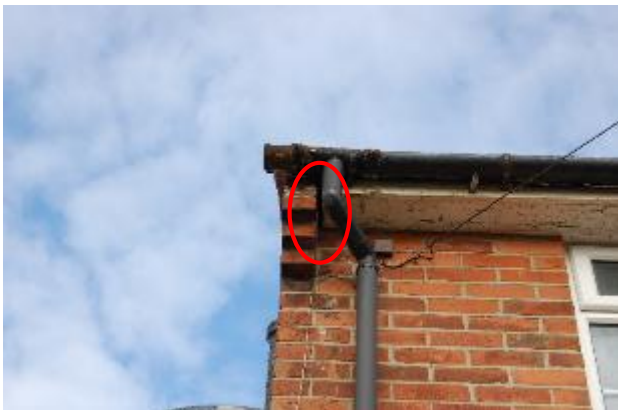
Photograph 5. A gap noted during the survey, between the wall and the boxed eaves (indicated by the red circle).
