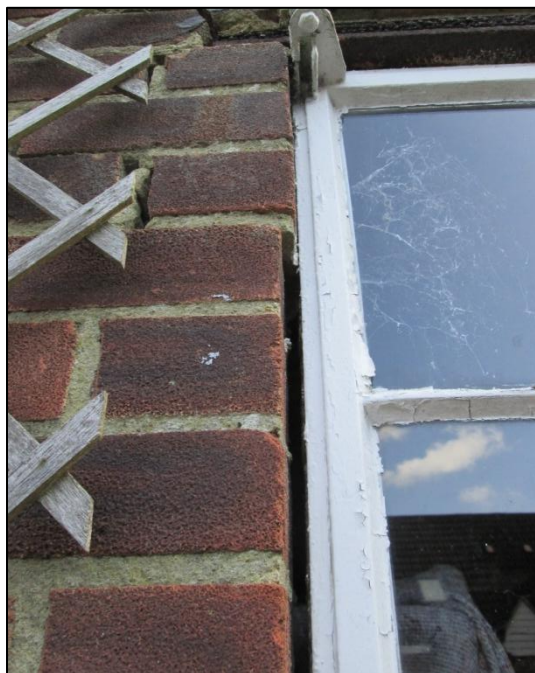
Figure 9 – gaps around windows due to structural issues
