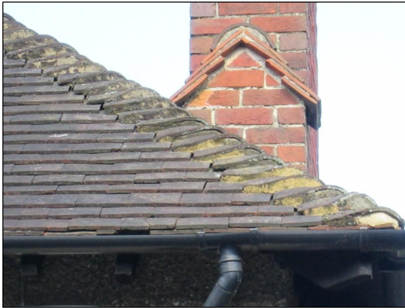
Figure 12 – Sections of mortar missing from the hips
