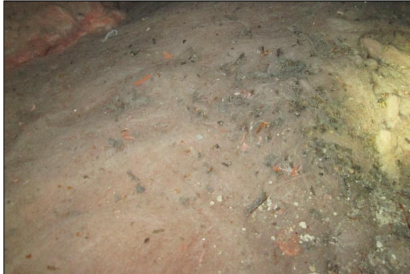
Figure 6 – collection of bat droppings underneath the ridge board
