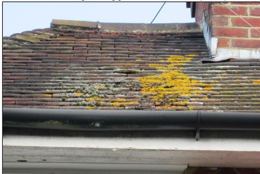
Figure 11 – Open ended tiles close to the eaves
