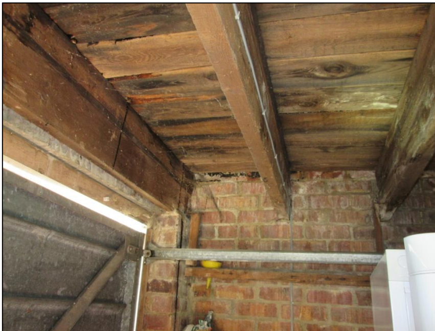
Figure 8 – shows interior of the garage which has a boarded flat roof, areas of damp and gaps which allow draughts
