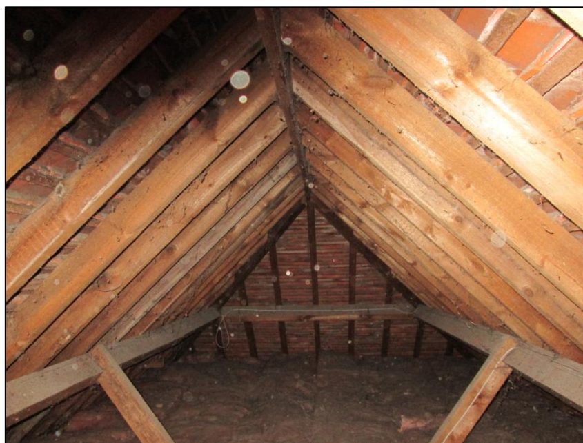
Figure 4 – Roof void showing lack of underlay
