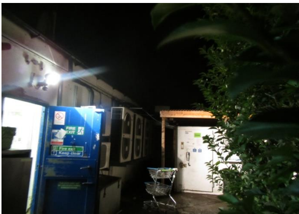
AC Units Mounted on Rear Wall
