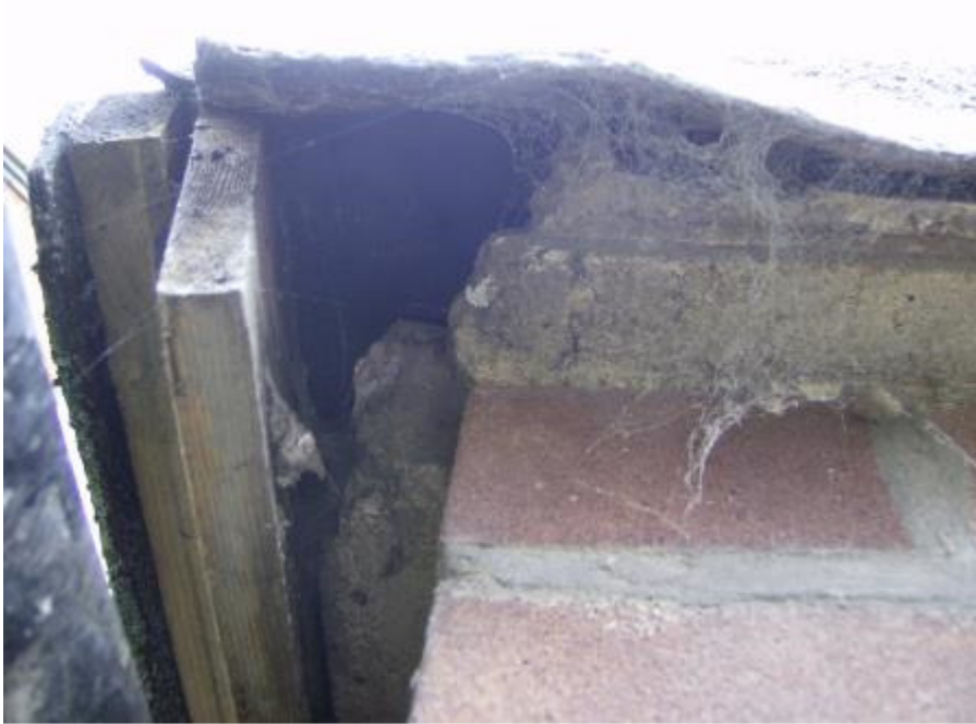
Photograph 5: Building 2 – hole between roofing and side wall, covered in dense cobwebs.
