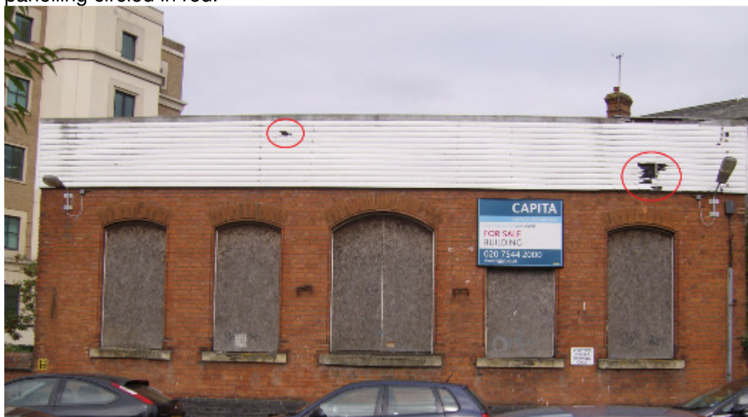
Photograph 2: Building 1 (Figure 1, Appendix A), southern wall with cavities in panelling circled in red.
