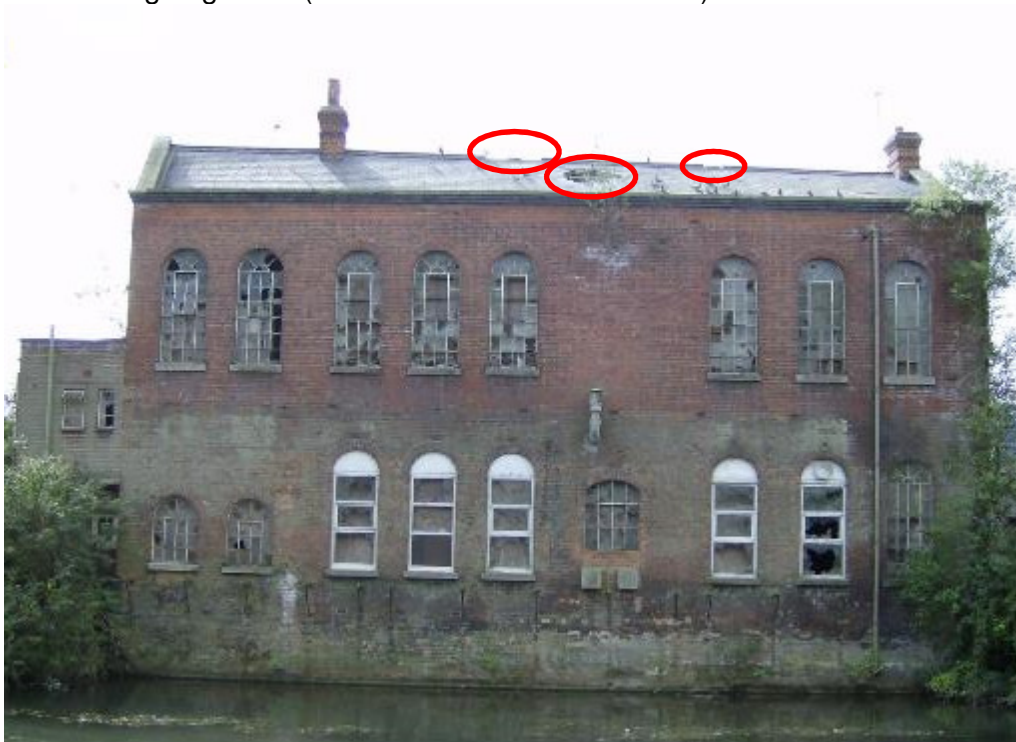
Photograph 7: Building 4 – northern view – with broken windows, a cavity into roof and missing ridge tiles (last two features circled in red).
