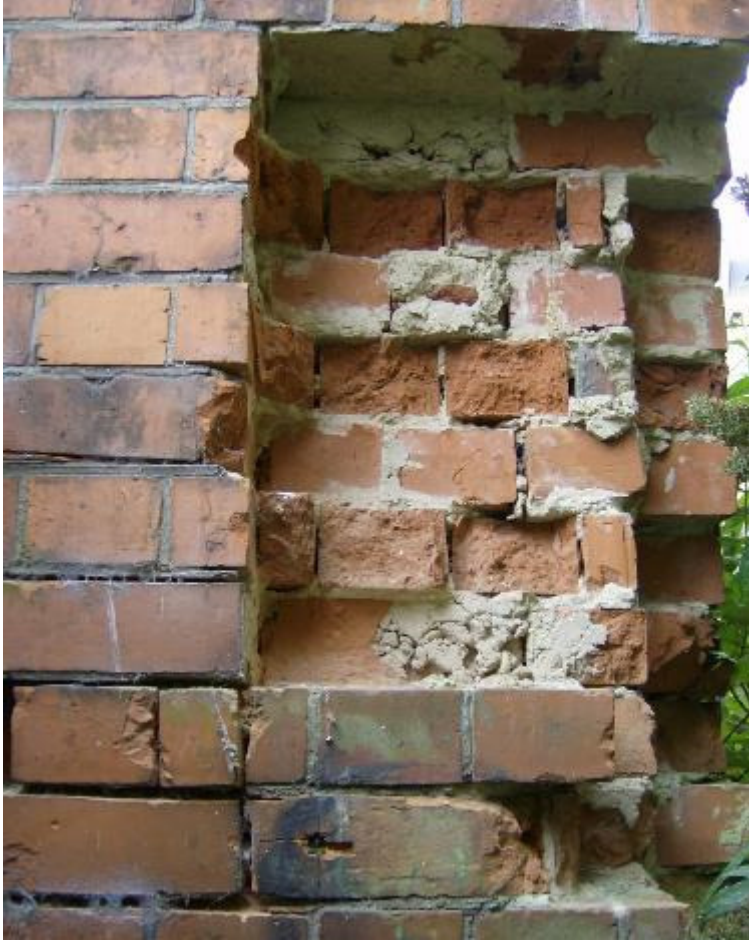
Photograph 3: Gaps in brickwork on eastern wall of B1.
