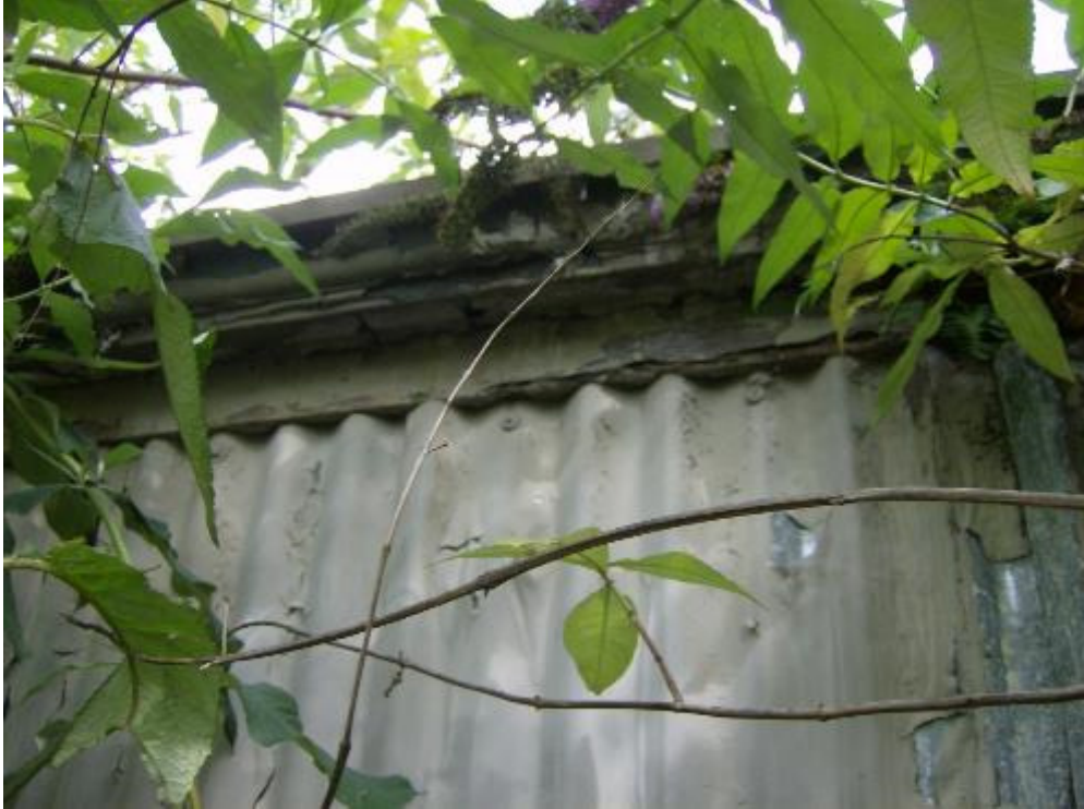
Photograph 9. Potential bat access point – gaps in rotten soffits and fascia boards.
