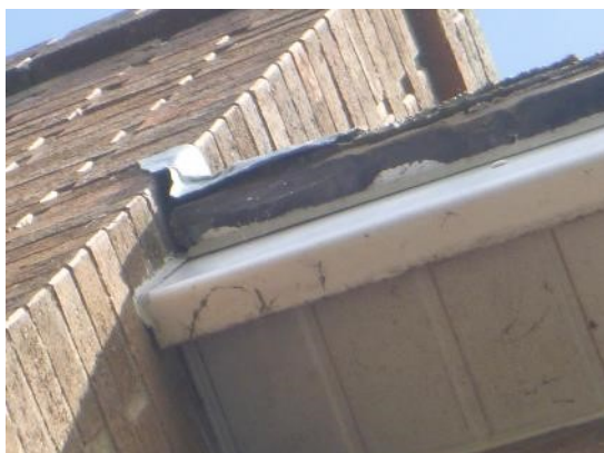
7. Superficial, slight gap under the lead flashing at the northern side of the chimney.
