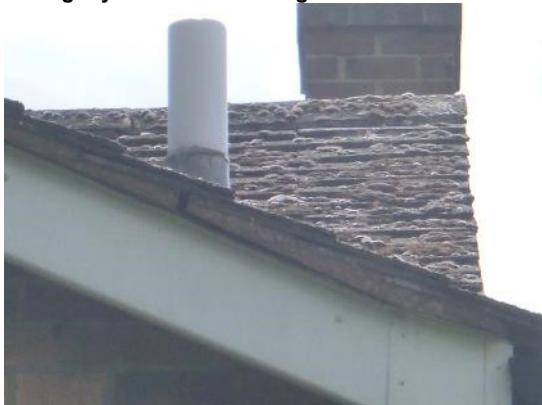
5. Crack in the mortar on the front gable end.
