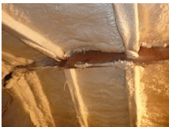
11. Ridge largely covered with the foam and cobwebbed.
