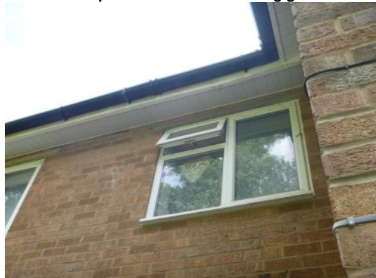
6. uPVC soffits tightly sealed to brickwork walls.
