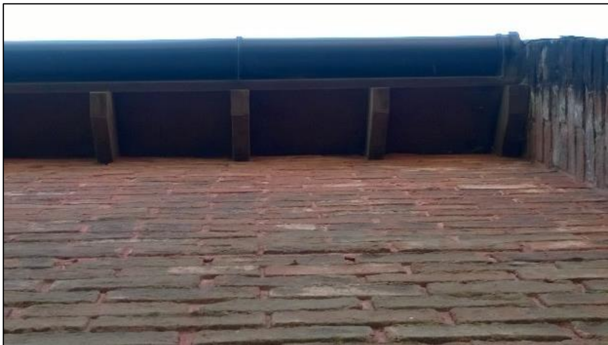
Photo 5: Timber boards protruding from loft.
