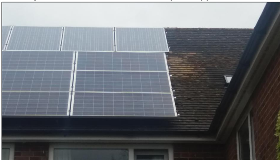
Figure 7 – Solar panels fitted on southern elevation
