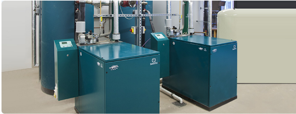
Figure 8: Example Mini-CHP Engines.
