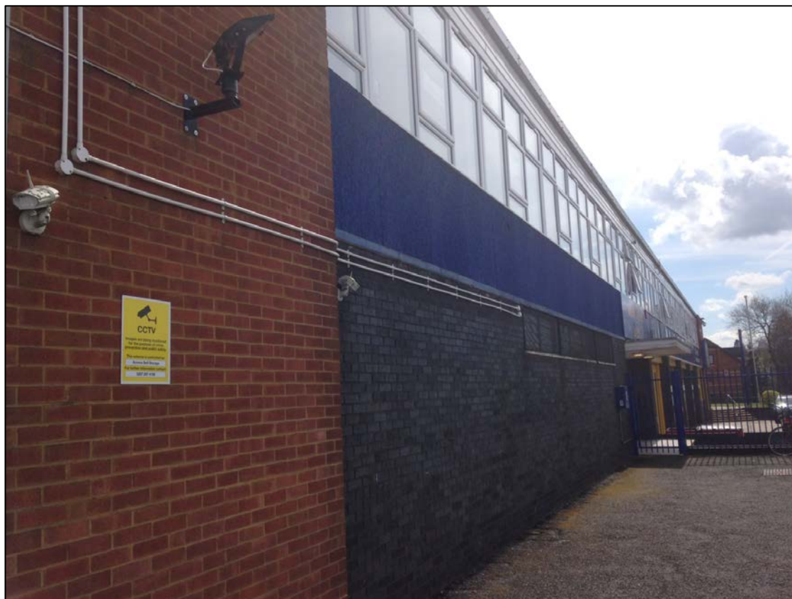
Photograph 1: Security lighting on eastern aspect of building. Photograph taken by Adam Earl 12/04/2016.
