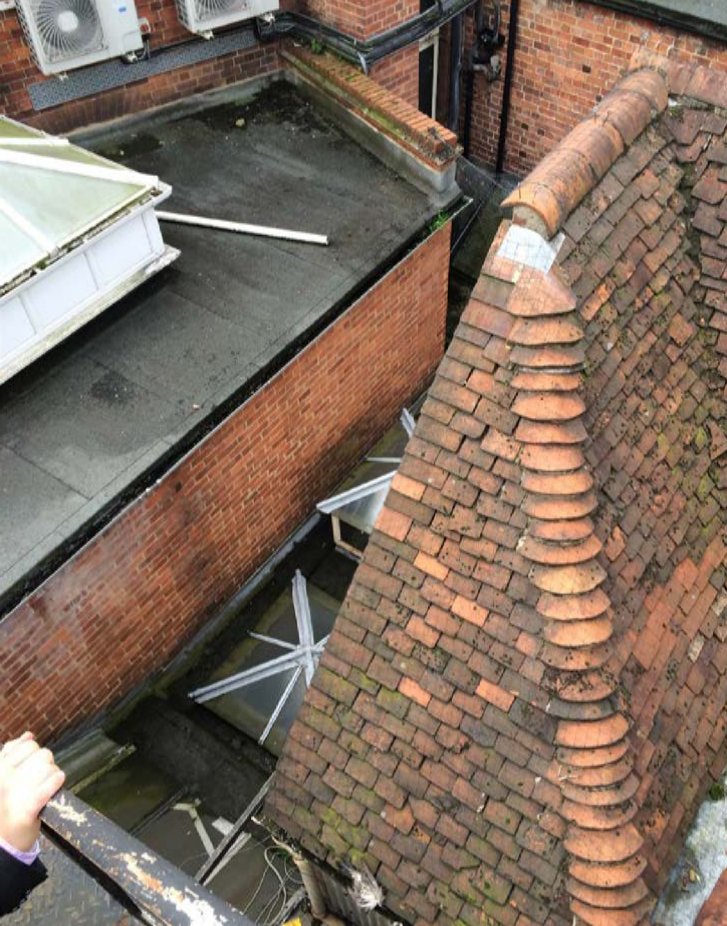
Fig 2.11: Various ad-hoc structures at rear of Jacksons
