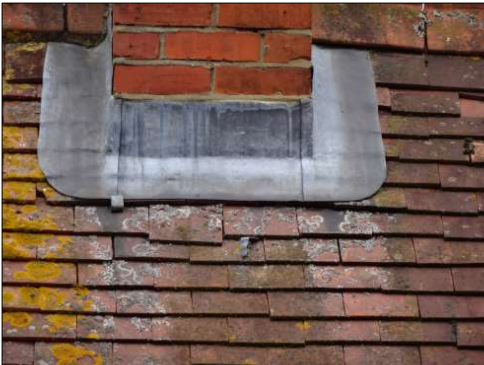
Figure 5. Example of gaps in lead lashing, 11 Darell Road, Caversham.
