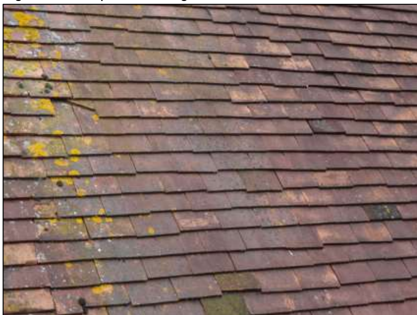
Figure 3. Example of missing tiles, 11 Darell Road, Caversham.
