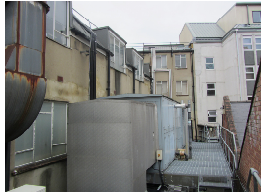
Existing air handling unit to be replaced
