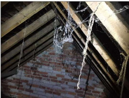
Photo 9 – Cobwebs to ridge (looking south east)
