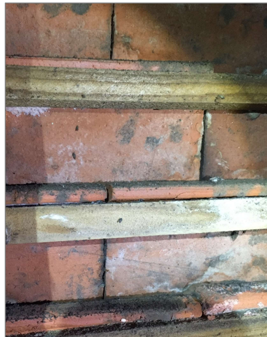
Photo 12 – Bat droppings to underside of tiles
