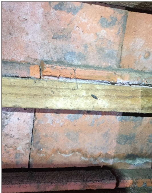
Photo 11 – Bat dropping to tile batten
