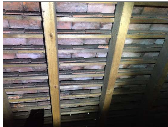
Photo 8 – Roof tiles unlined
