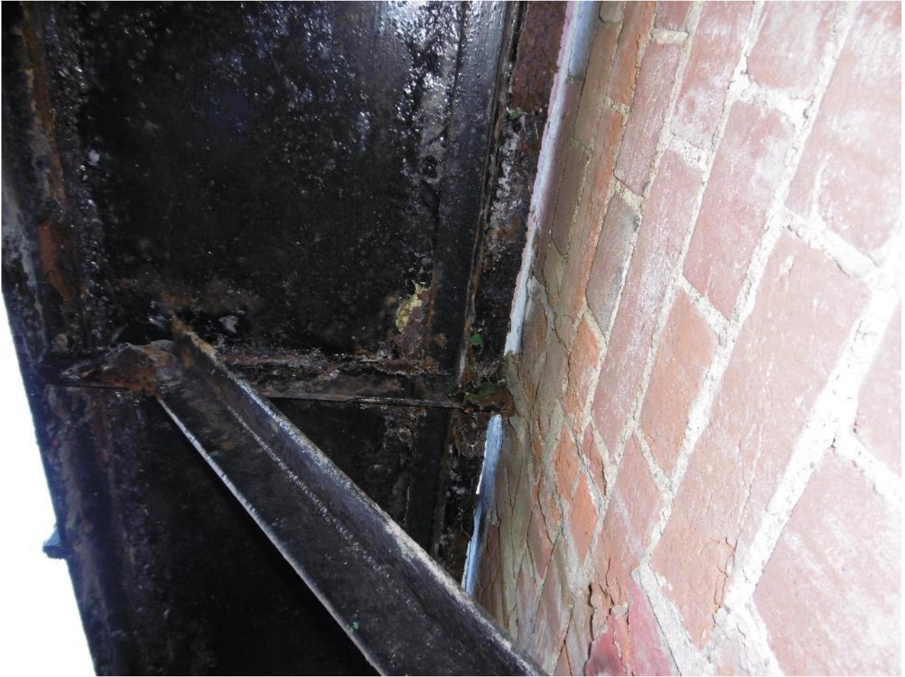
View showing corrosion
