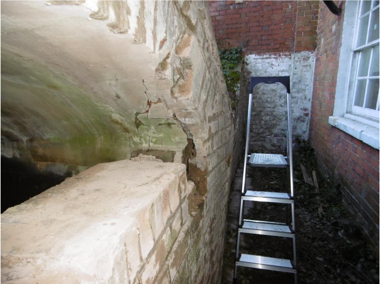
View showing movement of retaining wall
