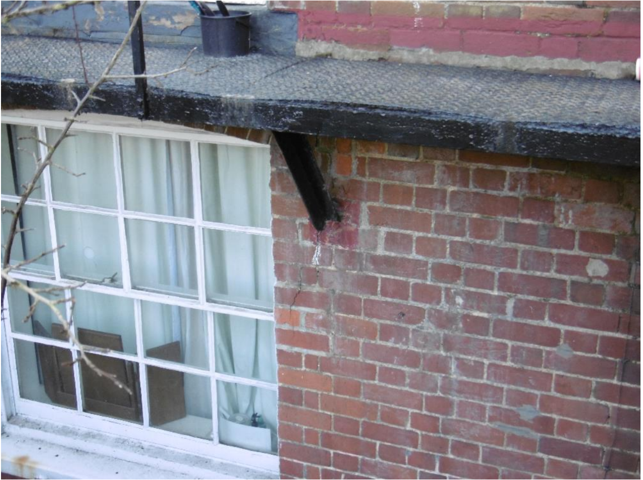
View showing damage to brickwork around bearing in wall
