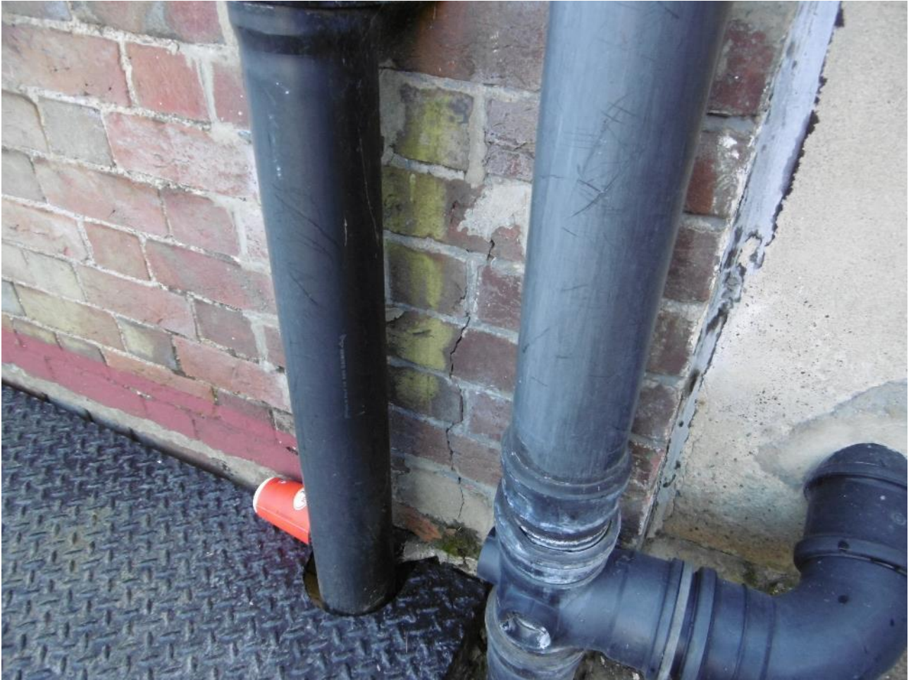
Cracking in brickwork
