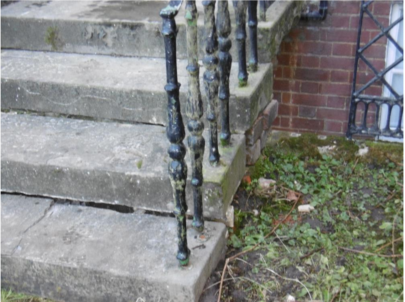
View highlighting movement of steps and deterioration/movement of brickwork and fill below.
