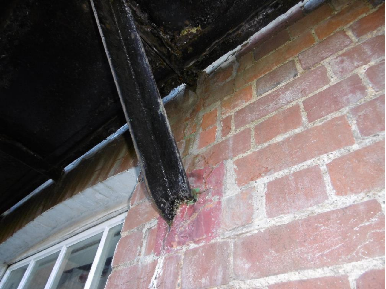
View on bearings in external wall – note damage to brickwork
