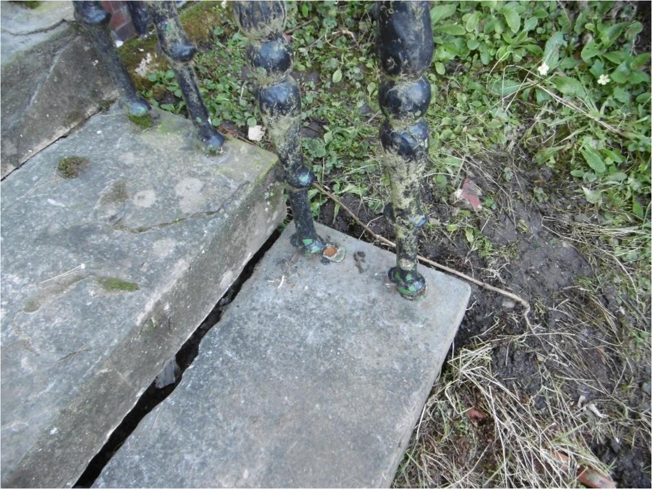
View showing movement of steps and failure of uprights.
