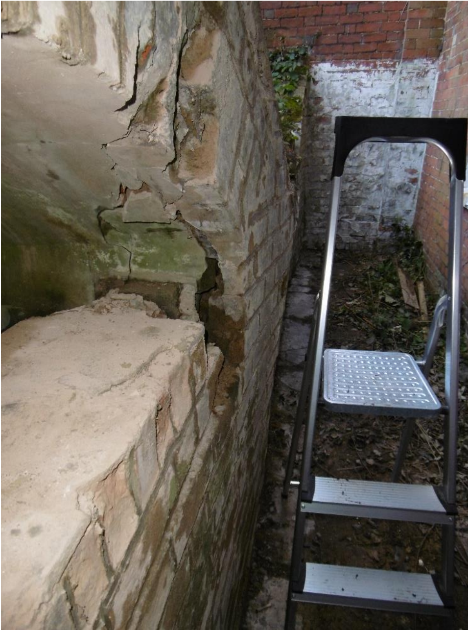
View showing movement of wall and damage to adjacent arch
