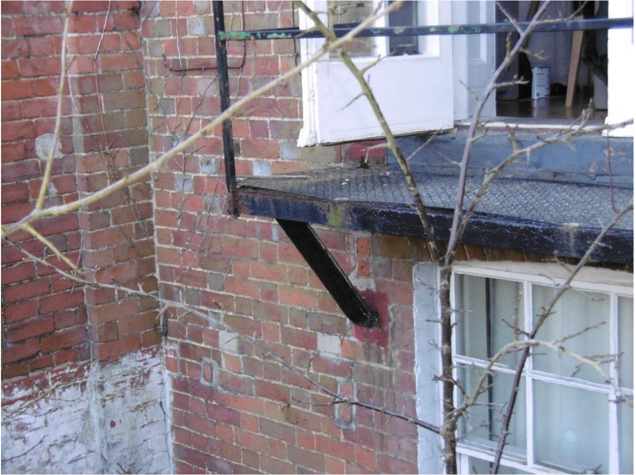
View highlighting corrosion of durbar plate in particular
