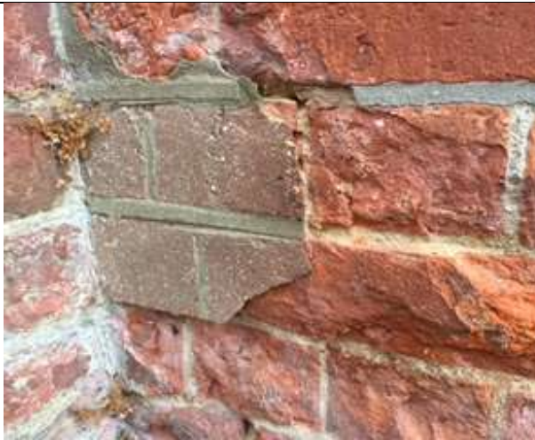
19 – Spalled brickwork that has blown the brick face
