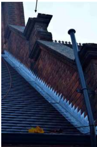
Hole in roof where brick hit and bounced off
