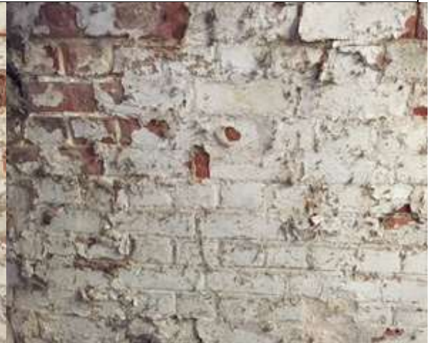
24 – Dampness to brickwork internally
