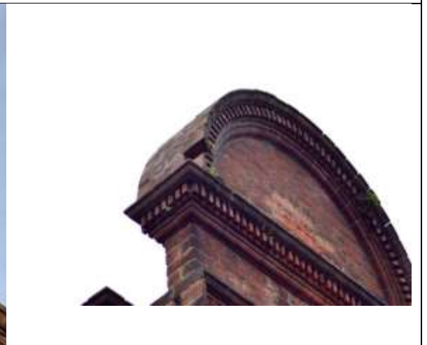
8 – Missing brickwork to high level gable parapet
