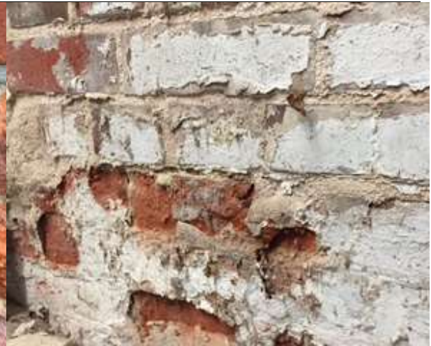
20 – Spalled brickwork increasing brick porosity
