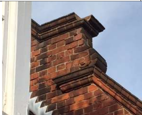
7 – Brickwork already fallen from high level
