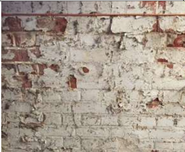
23 – Dampness to brickwork internally
