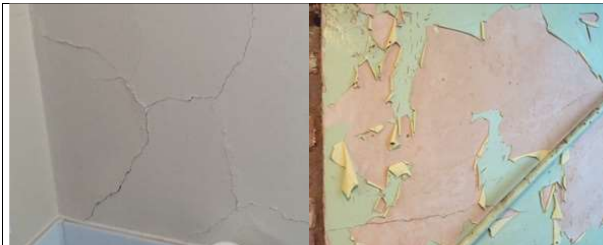
29 – Damaged plaster from water ingress
