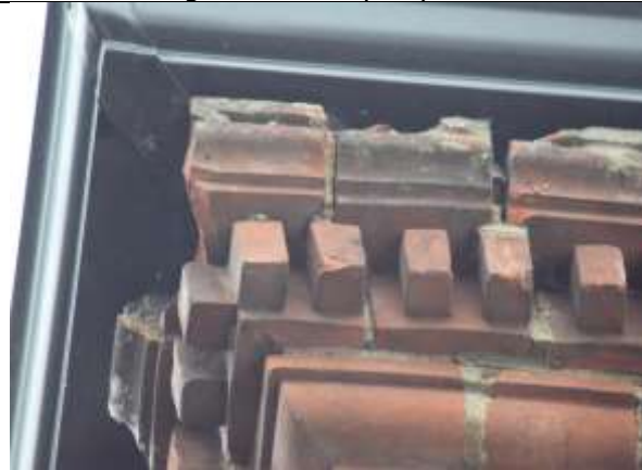
5 – Brickwork at high level about to fall
