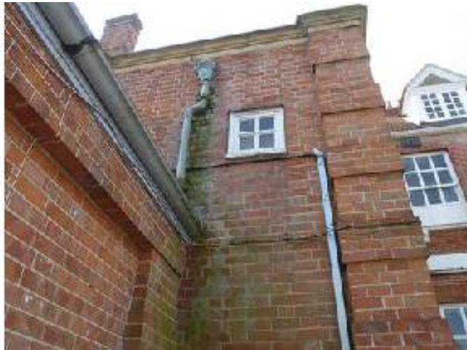
REPAIRS TO RAINWATER GOODS REQUIRED
