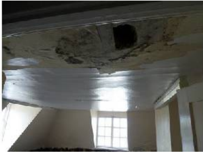
CEILING IN CLASSROOM 01 TO BE REPAIRED OR REPLACED
