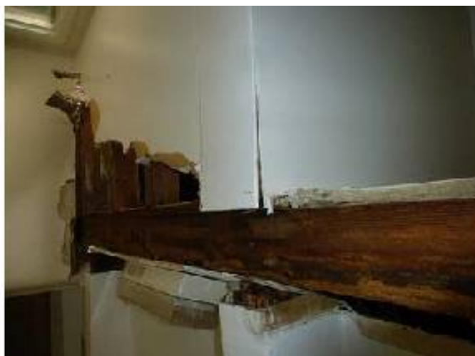
PLASTERWORK TO BEAM REQUIRED
