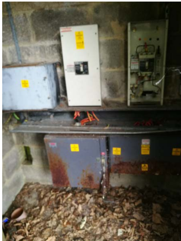
Plate 18 – View inside the electricity book on site
