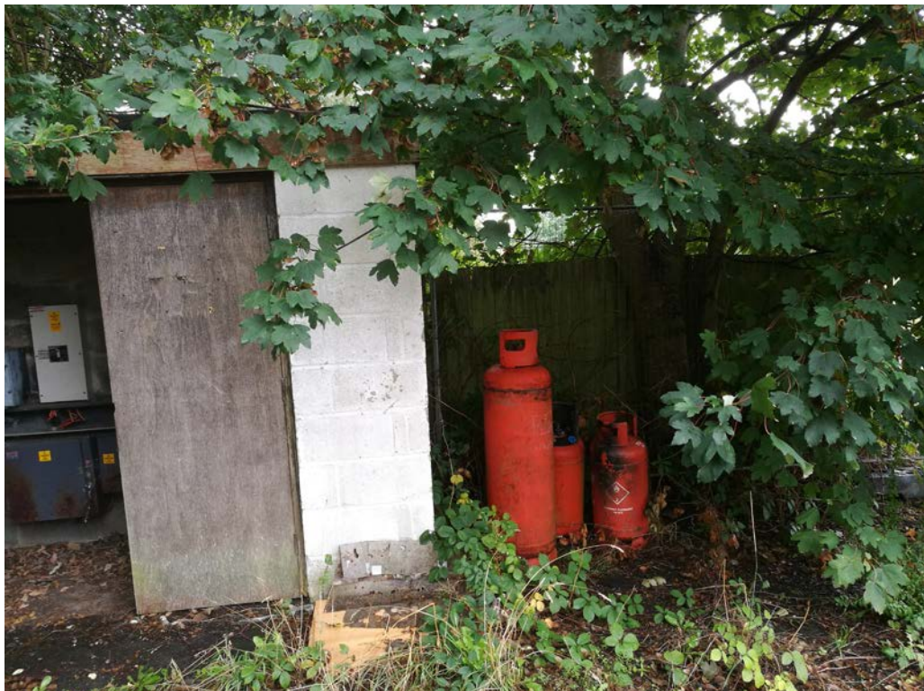
Plate 14 – Evidence of disused gas canisters on the site
