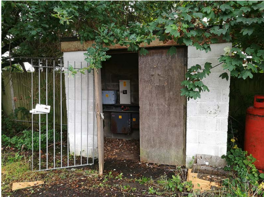
Plate 13 – Electricity box located on the south boundary of the access road into the site
