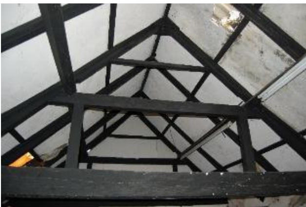
Photograph 3. The plaster board on the ceiling of the upper room in Building 1 (southernmost end)
