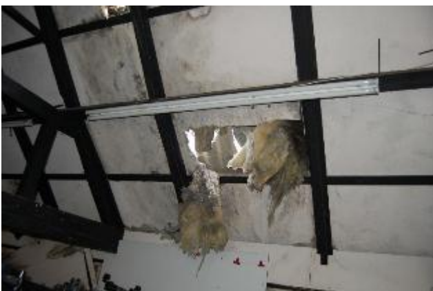
Photograph 5. An example of a hole noted within the plaster ceiling and asbestos sheeting of the roof.
