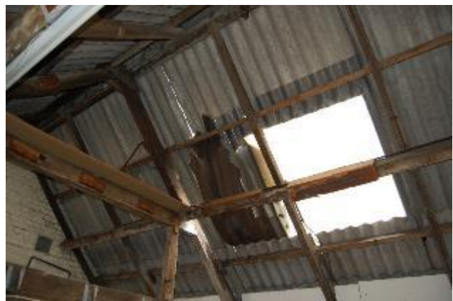
Photograph 4. The northern end of the upper room of Building 1, note there is not plaster board cover to this end.
