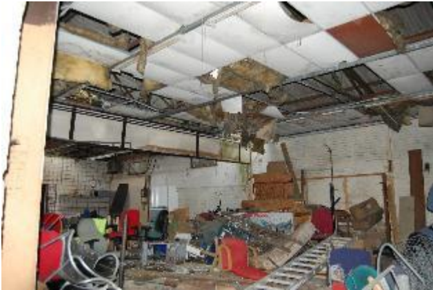
Photograph 13. The partial false ceiling in Building 2, only a small number of panels remain.
