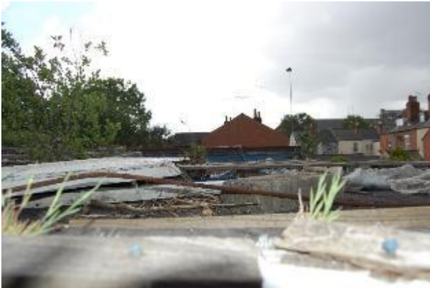
Photograph 25. The poor repair of the roof of Building 5.
