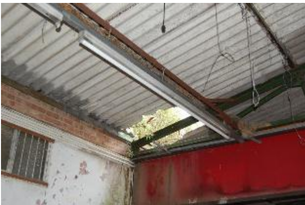
Photograph 11. An example of one of the many holes within the asbestos sheeting of the roof of Building 2.
