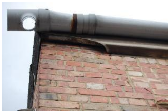
Photograph 6. Broken end of the asbestos that is moulded over the top of the wall, creating a bargeboard like feature.
