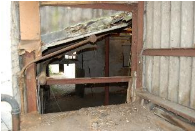
Photograph 21. Photograph showing the large gap within the interior wall of Building 4, leading into Building 3.
