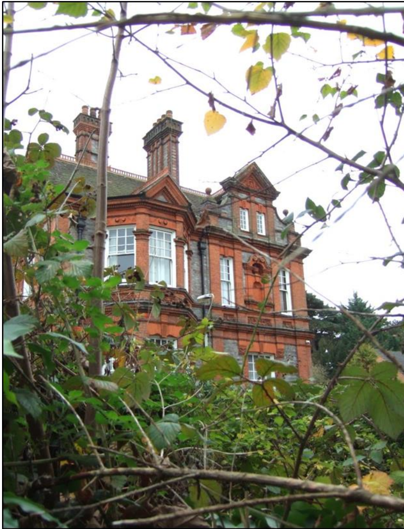
Figure 20 The ornate North elevation obscured by undergrowth. Gaila Adair 2016
