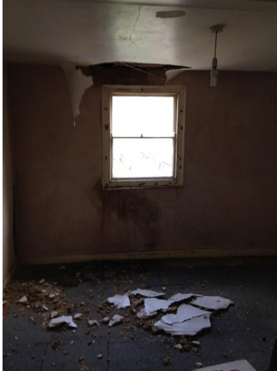
005 – Dilapidated state of first floor
