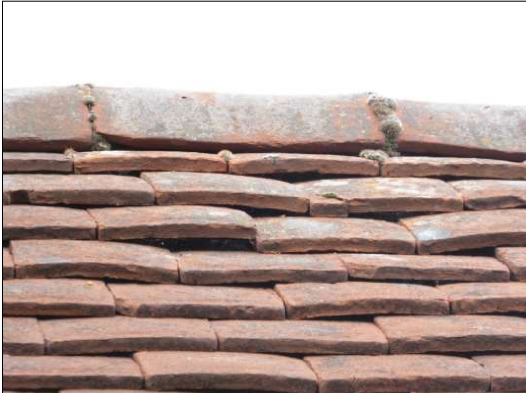
Figure 6. Example of gaps under tiles. Henley Road Cemetery, Caversham. 03.07.17
