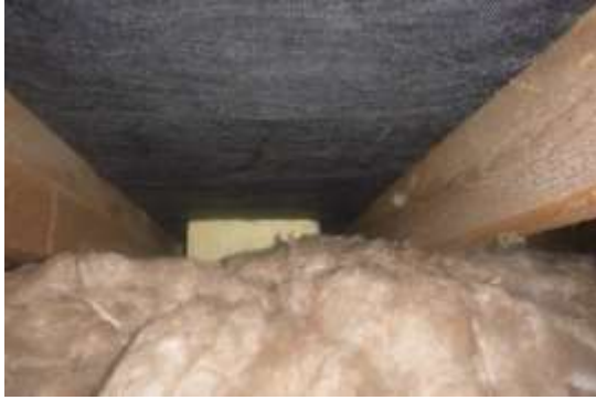
9. Gaps at eaves where the fibreglass does not fit tightly.
