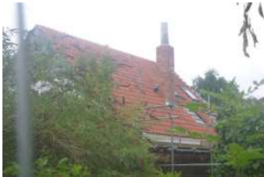
3. Missing areas of tiles to the side of the property and lifted lead flashing around the base of the chimney.
