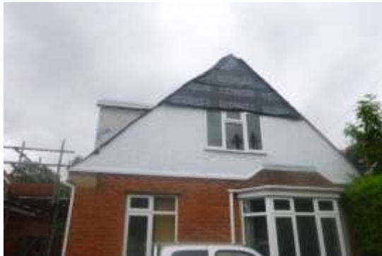
1. Front view of the house showing the removed timber cladding at the front of the property.
