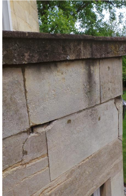
Photo 2 – Deteriorated cramps and loose stonework to single storey bay window on the South elevation.
