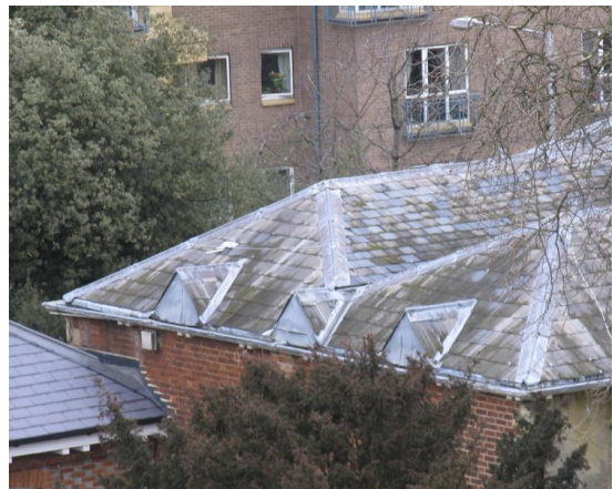
Photo 4 – Stained, slipped and slipped tiles to the West elevation.
