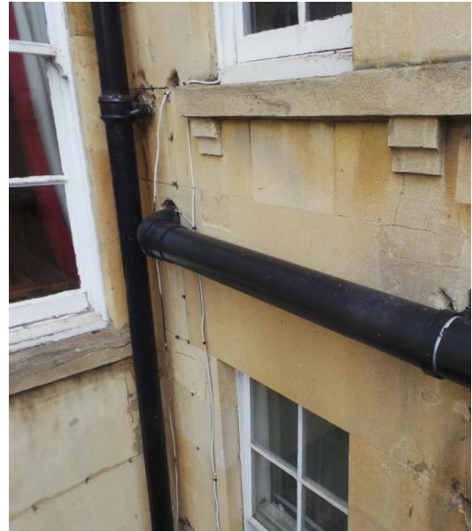
Photo 6 – Corrosion of downpipe bracket and staining to stonework cladding
