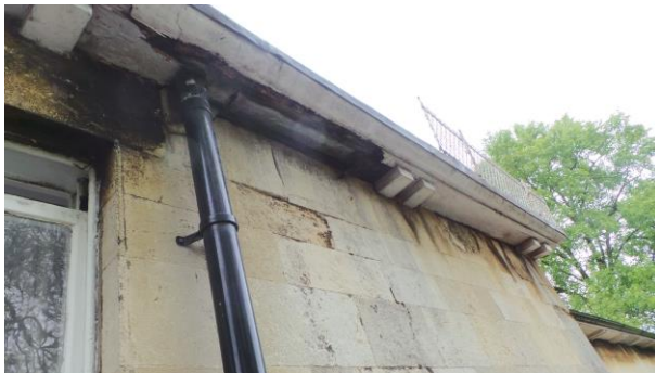
Photo 7 – Deteriorated timber soffit detail. Lead linings are located to the upper edge.
