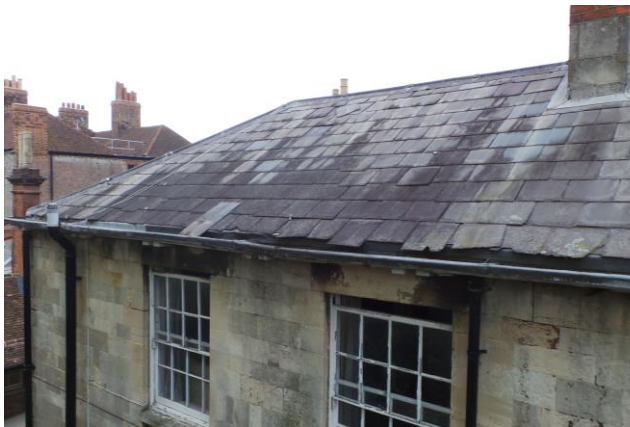
Photo 3 – Slipped, cracked and broken roof tiles to the South elevation of the West wing.
