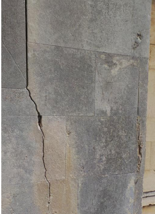
Photo 1 – Vertical crack to the South Elevation
