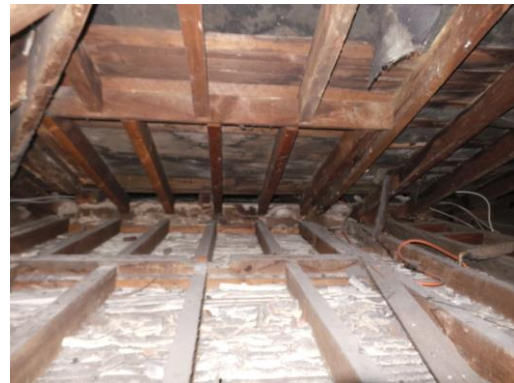
Photo 8 – Lack of thermal insulation to roof void. Lathe and plaster ceiling visible to West wing roof void.
