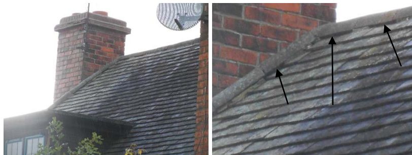
Plate 3.4: Missing mortar under ridge tiles
