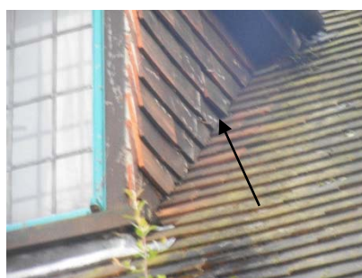
Plate 3.5: Gap under the dormer window hanging tile
