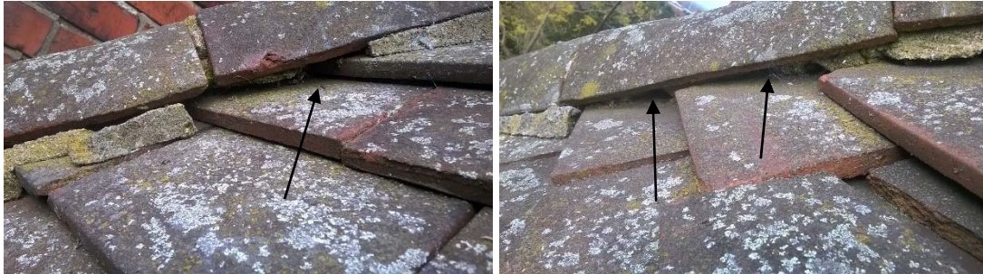
Plate 5: Gap under the ridge tile with limited suitability for bats
