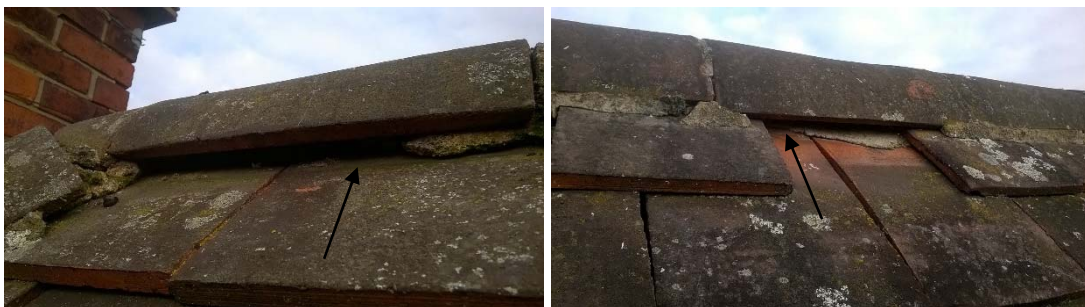
Plate 6: Gap under the ridge tile suitable for bats
