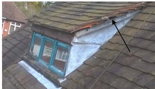
Plate 9: Suitable cavity for bats under the dormer window roof tile
