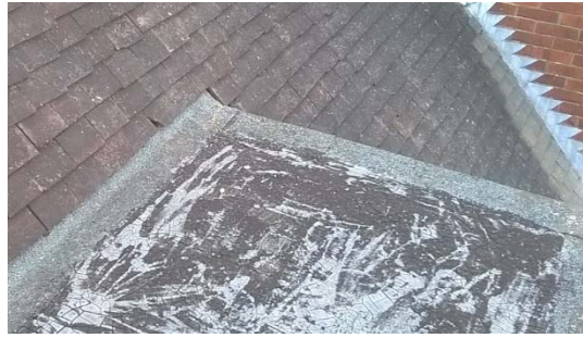
Plate 7: Broken tiles around the dormer windows
