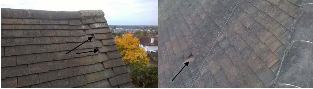
Plate 3: Missing/gappy roof tiles
