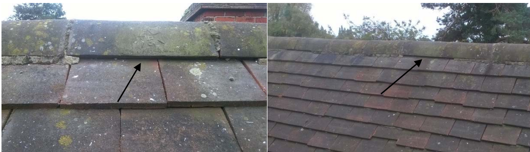
Plate 4: Mortar missing under the ridge tile but no suitable gaps present
