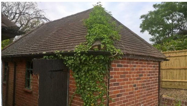
Plate 4.5: Example of Damaged/Lifted Tiles
