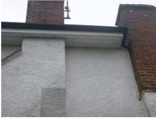
7. The narrow gap behind the soffit box on the eastern elevation.
