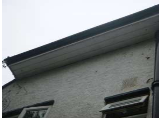
8. The narrow gap behind the soffit box on the western elevation.
