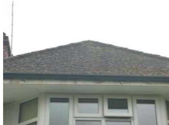
4. Intact mortar under the hip tiles.
