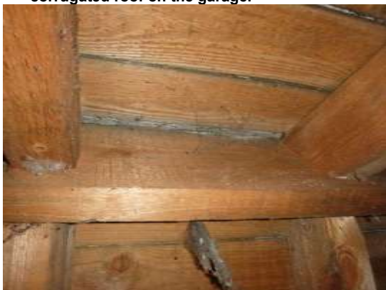
11. Part of the uninsulated floor and open eaves.
