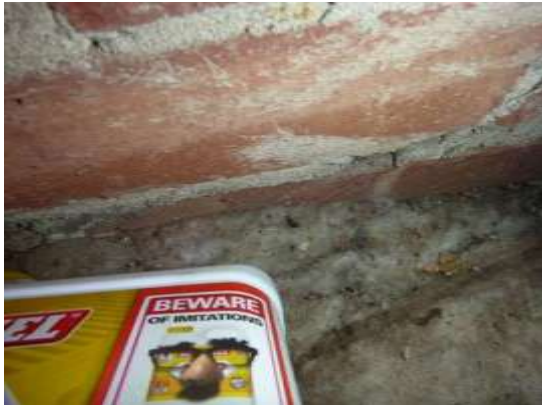
15. One of the bat droppings at the western end of the roof space.
