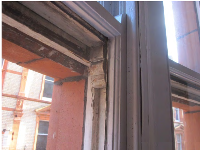
Rot on front sash windows
