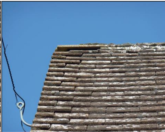
Photograph 4: Gaps within the mortar of the ridge at the gable end to the west of the property.
