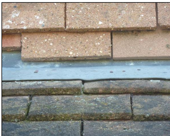
Photograph 6: Droppings recorded on the lead flashing beneath a roof dormer window on the rear elevation.
