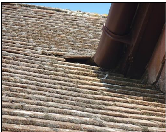
Photograph 5: Gaps between hanging tiles by the valley meeting point to the rear of the north facing property.
