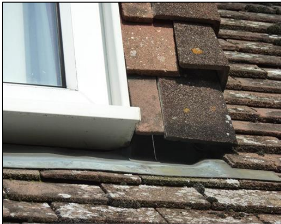
Photograph 3: Gaps beneath hanging tiles around the roof of the property.
