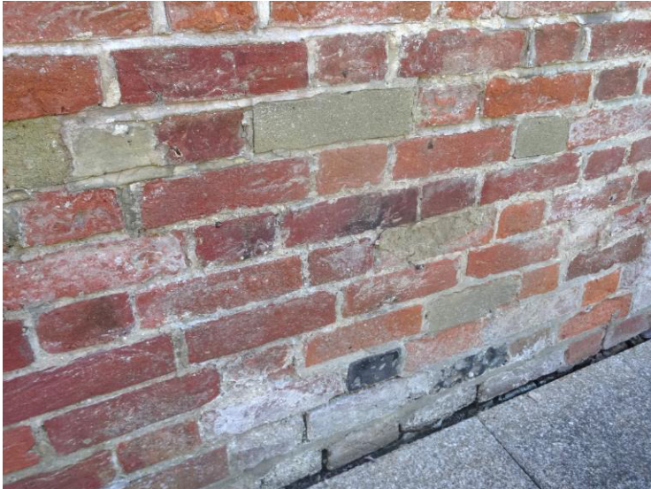
25. Rear elevation: Facing of rendering on spalled bricks.
