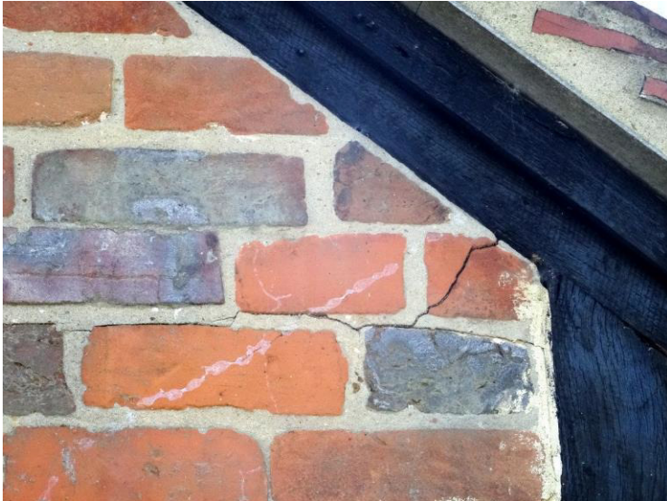
17. North elevation: Cracks in brickwork joints and through brick
