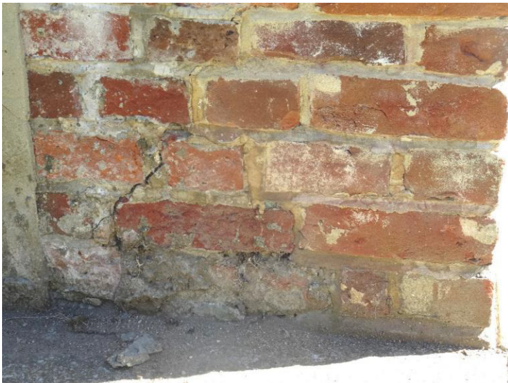
22. Rear elevation: Diagonal crack at south west corner.
