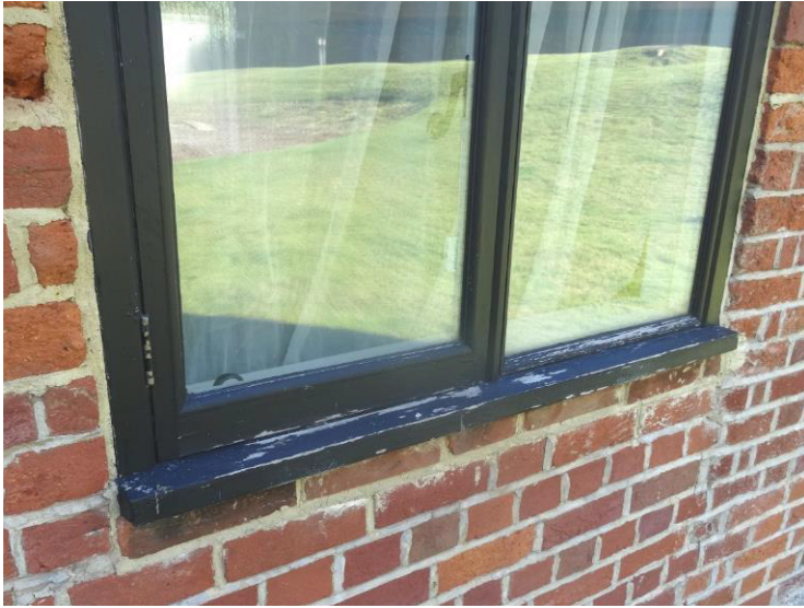
5. External paintwork in poor condition with bare wood exposed.
