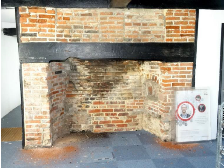
27. Open Plan Area: Spalled bricks in fireplace.
