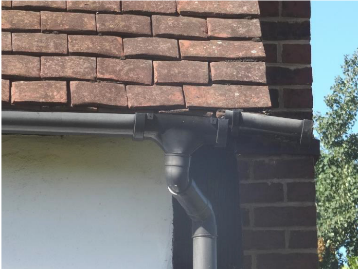
9. Front elevation: Detached gutter at north end.
