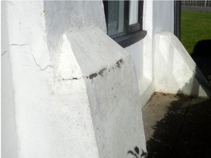
11. Front elevation: Horizontal crack with moss growth on buttress.
