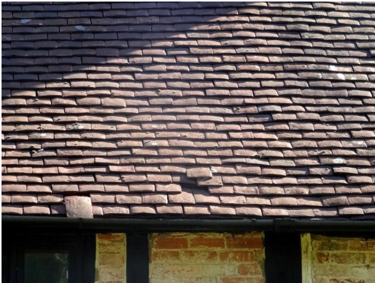
18. Rear elevation: Slipped and missing roof tiles.
