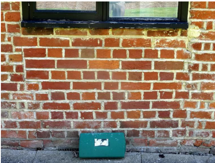
20. Rear elevation: Vertical cracks at window apron.
