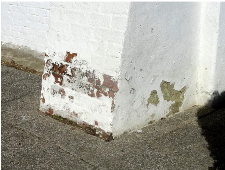
8. South elevation: Damp affected paint and detached rendering on buttress.
