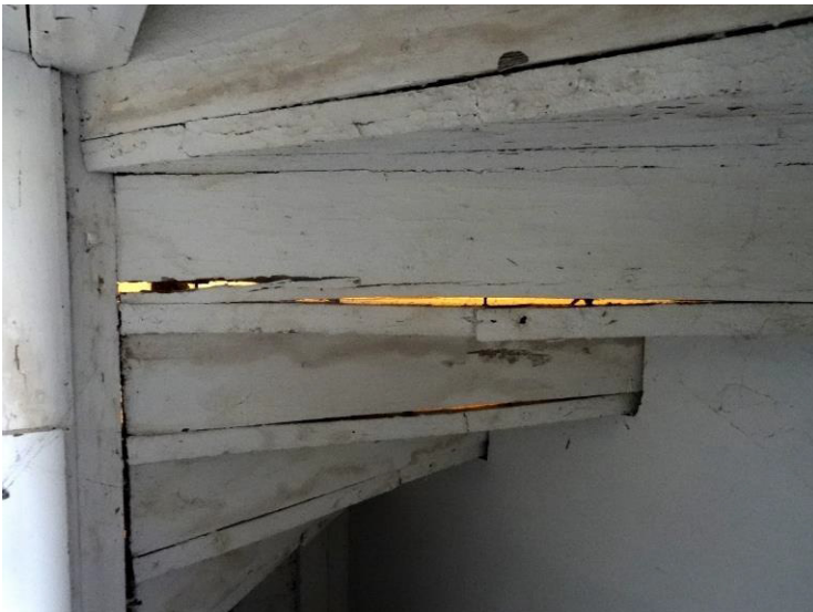
32. Staircase: Splits in timber and treads deflected.
