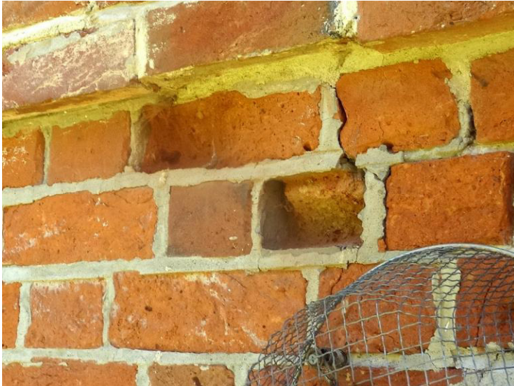
23. Rear elevation: Spalled bricks. Spalling exacerbated by the use of impermeable hard cement mortar, also cracked and detached.
