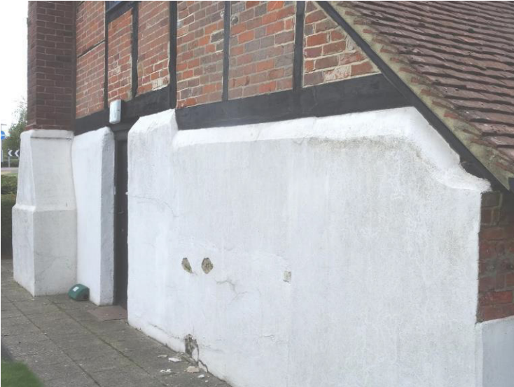
15. North elevation: Rendering cracked, hollow and detached in patches.
