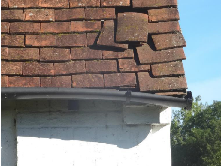
7. Slipped verge tiles and dropped gutter.
