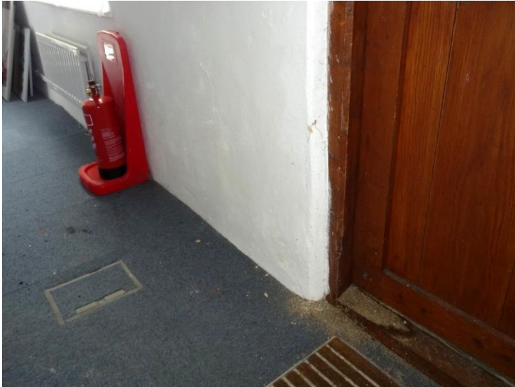
29. Open Plan Area: Detached plaster and dampness at front entrance door.
