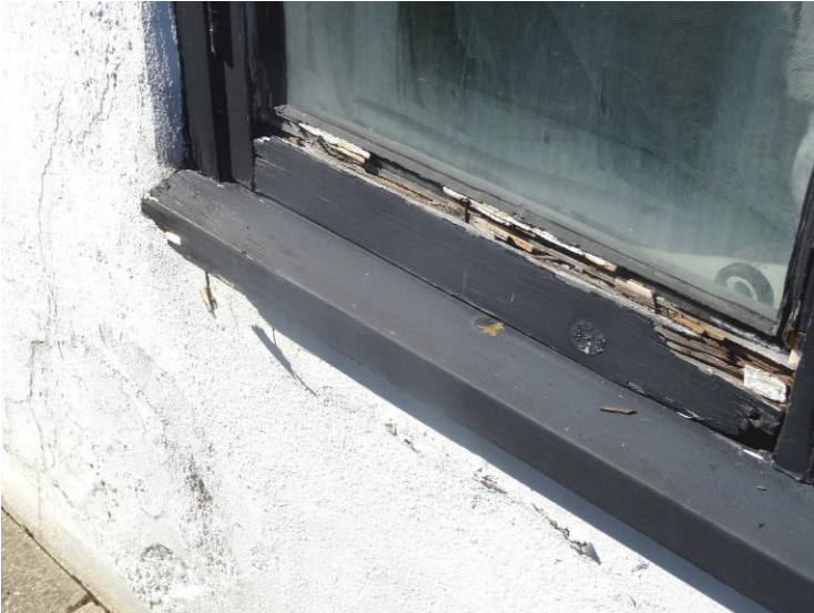
13. Front elevation: Reception room window rotten
