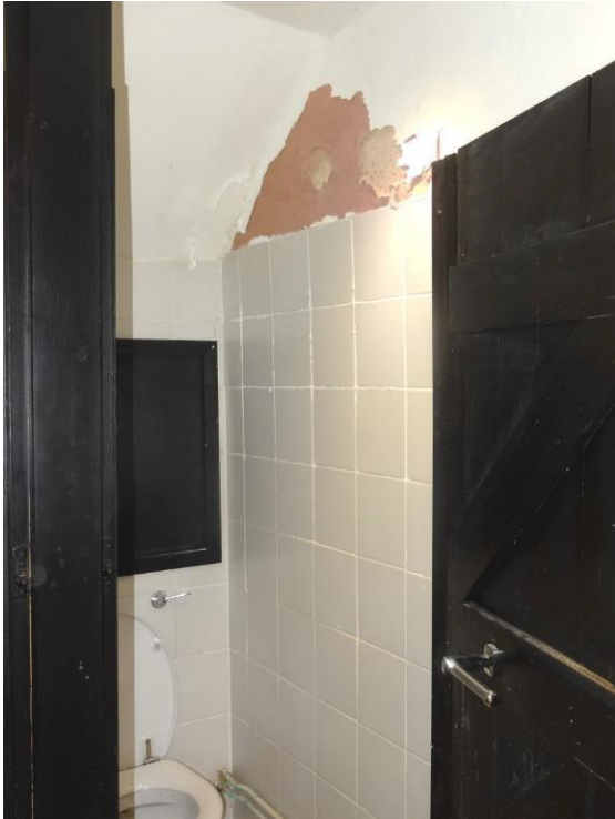
31. Ladies Toilet: Dampness and detached plaster and paint. Hollow wall tiles.
