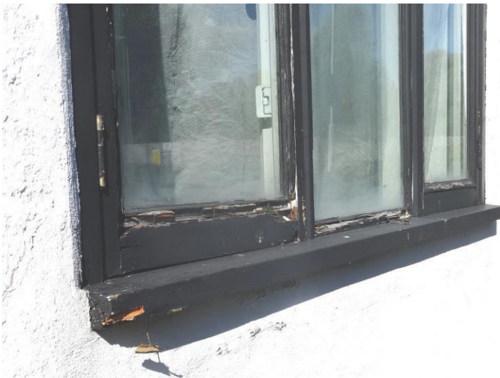
12. Front elevation: Reception room window rotten
