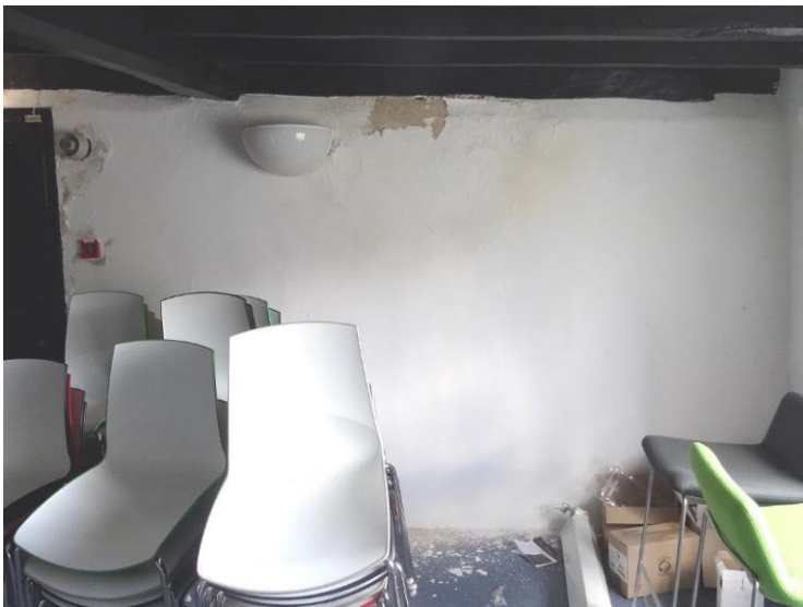
30. Open Plan Area: Detached surface plaster, cracked paint film and dampness on north wall.
