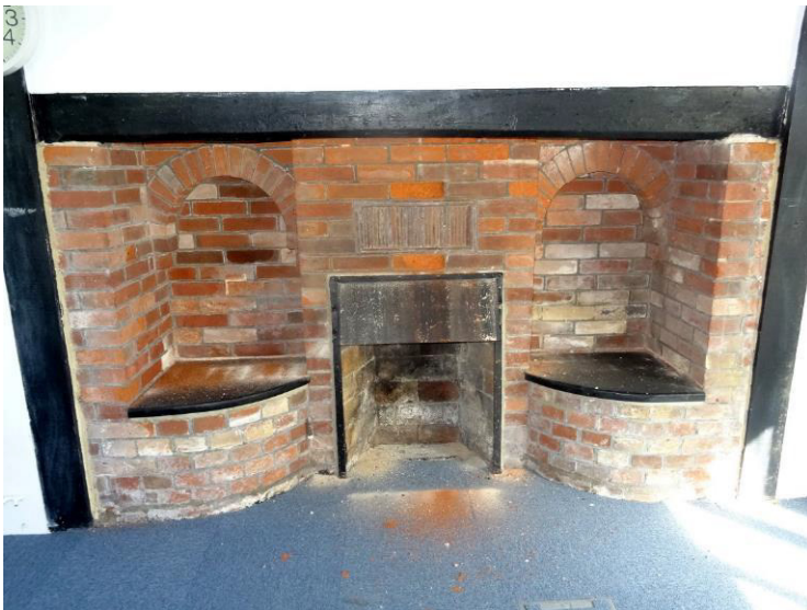
26. Reception room: Spalled bricks in fireplace.
