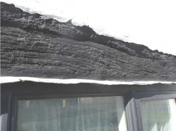
14. Front elevation: Timber frame degraded and crumbling.
