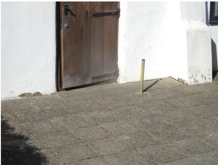
10. Front elevation: Dampness in wall at ground level.
