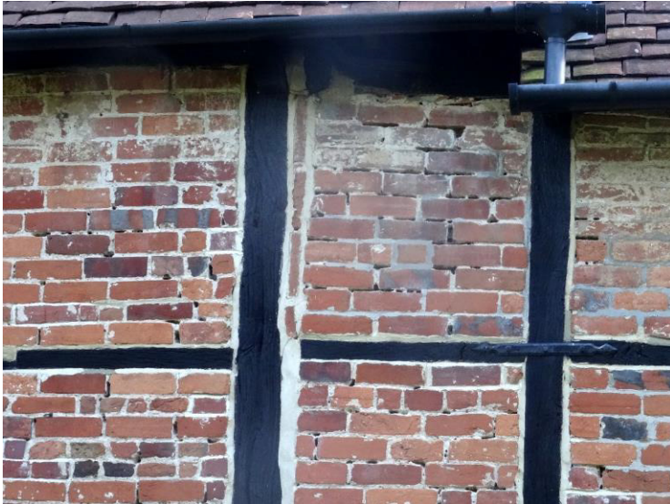
19. Rear elevation: Open joints in brickwork in timber framed panels.
