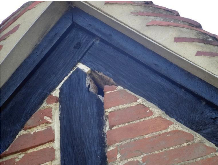
16. North elevation: Hole at ridge.
