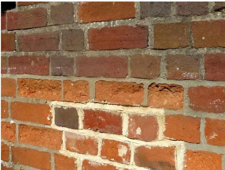
24. Rear elevation: Spalled bricks and patch of recently replaced bricks.
