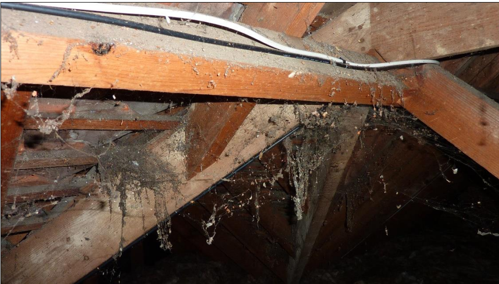
Figure 6 – showing high level of cobwebbing at 154 St Peters Road
