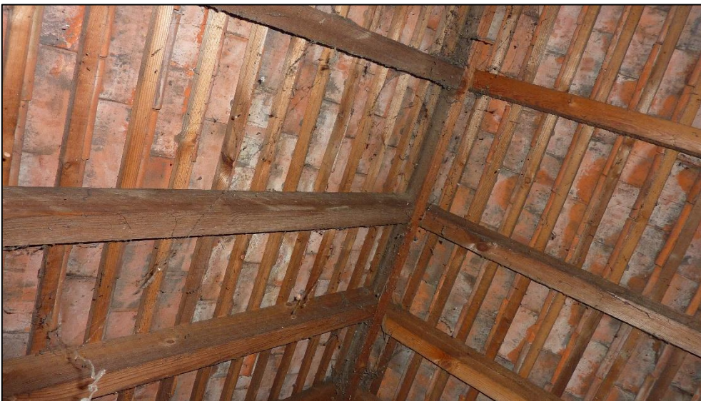
Figure 5 – showing lack of underlay interior of roof void at 154 St Peters Road
