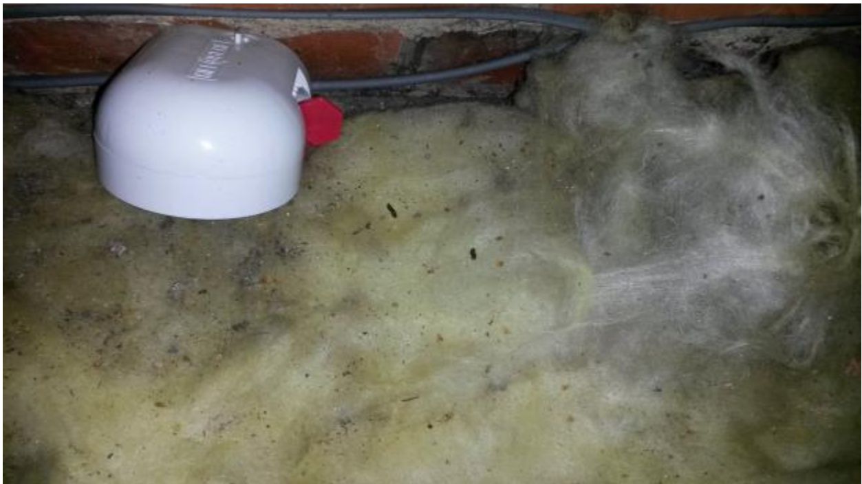
Photo 8: bat droppings below joining wall.
