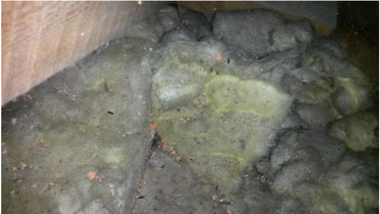
Photo 11: bat dropping scattered under the ridge of the bay window area.
