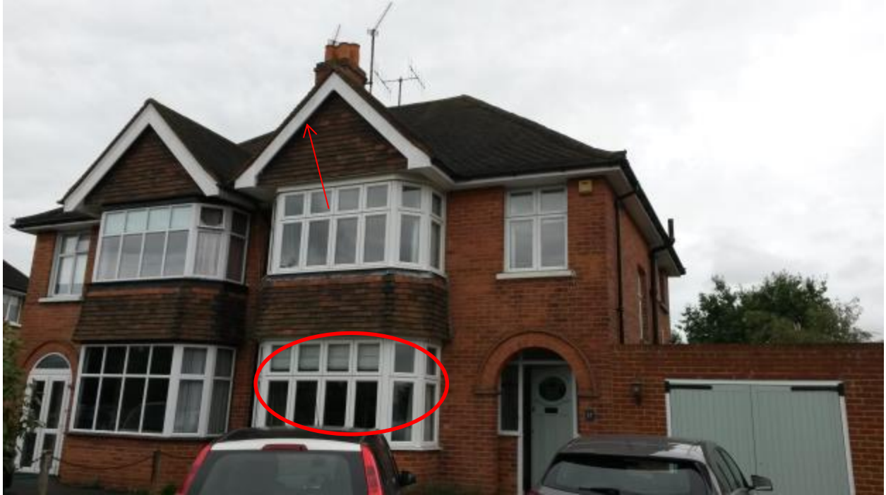
Photo 1: front of B1, western elevation. Location of bat droppings circled. Access point into loft shown with an arrow.
