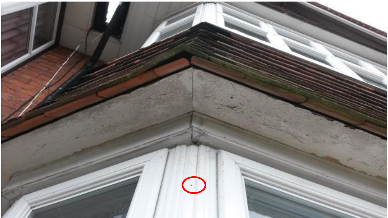
Photo 2: gap under hanging tile on the front bay window with a bat dropping directly beneath it.
