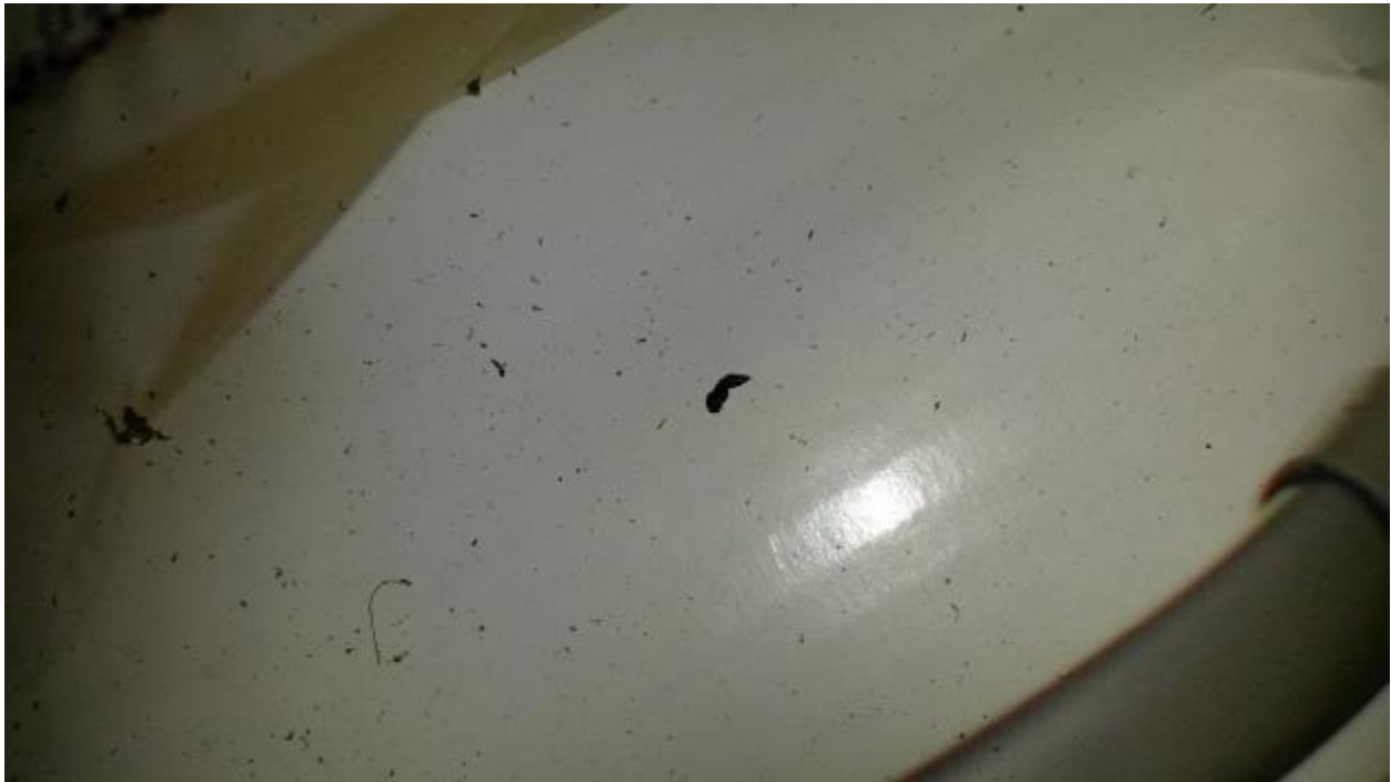
Photo 7: bat dropping in central loft space below the ridge.
