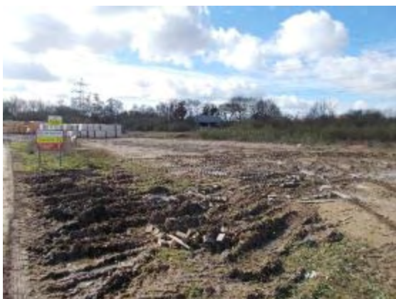
Plate 5. Disturbed bare ground from construction works
