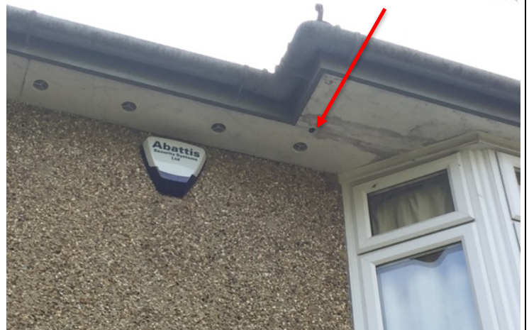
Photo 7 – Hole in soffit box – northern elevation
