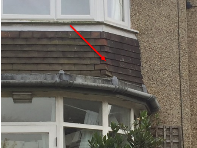
Photo 6 – Lifted hanging tiles – northern elevation
