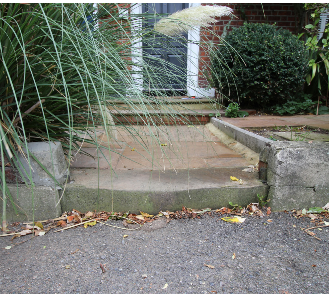
Existing low cement rendered walls.
