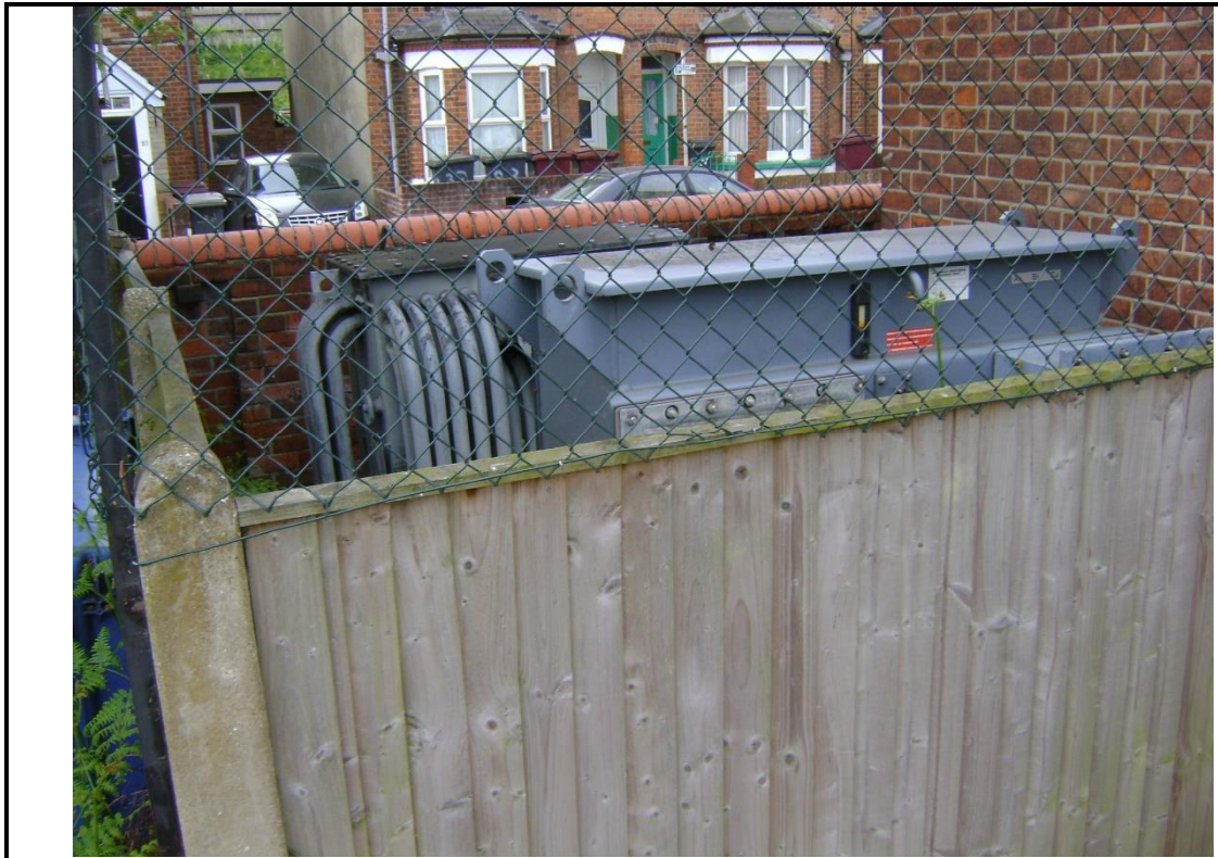
Photograph 3: Electricity sub-station in south.
