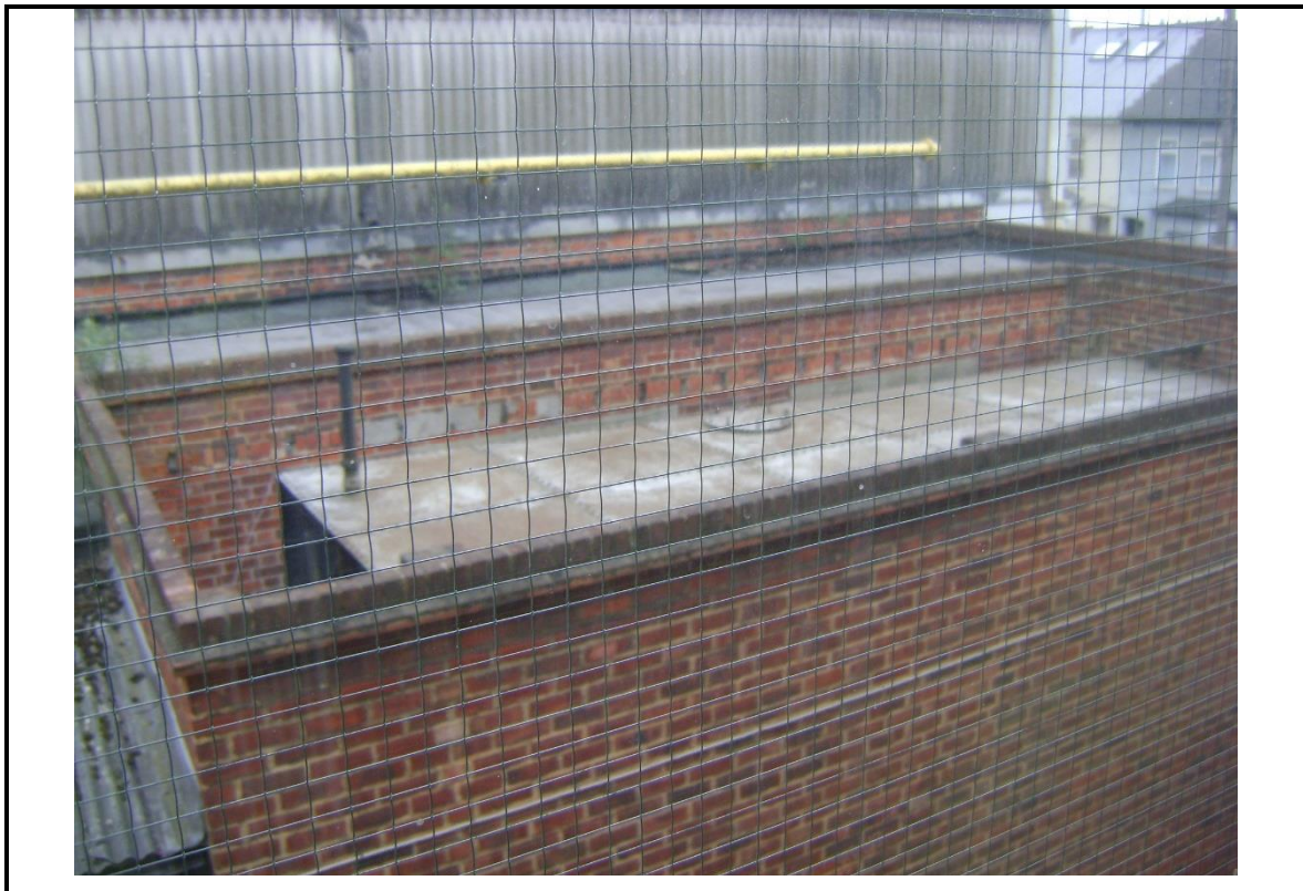
Photograph 5: Diesel Storage Tank.
