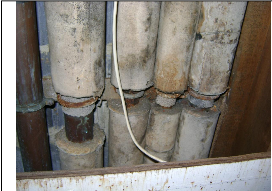
Photograph 7: Possible ACM cladding on First Floor.
