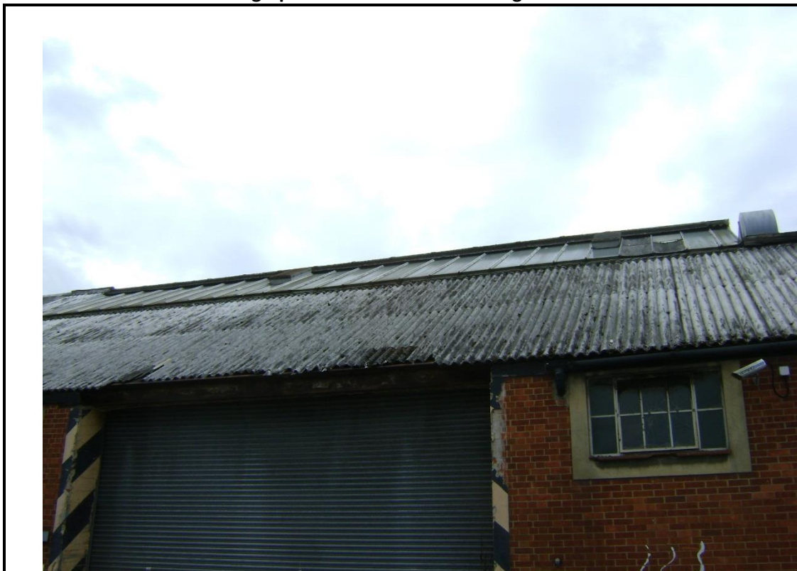
Photograph 8: Probable ACM roofing on northwest of main building.
