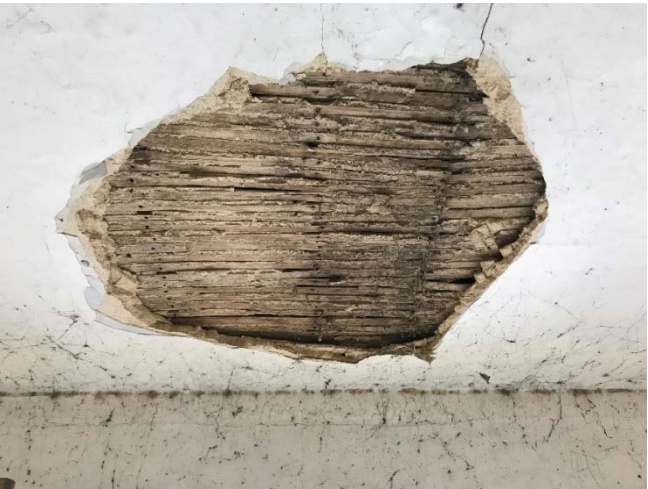
Figure 1: Area of missing / fallen plaster viewed with live plaster surrounding.
