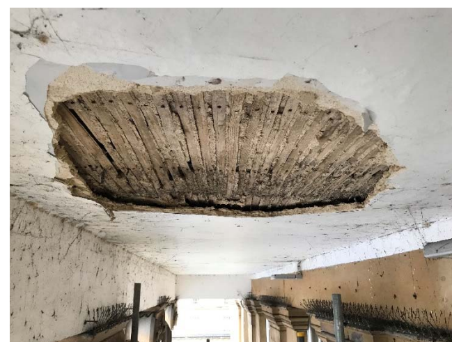
Figure 8: Area of damaged plaster
