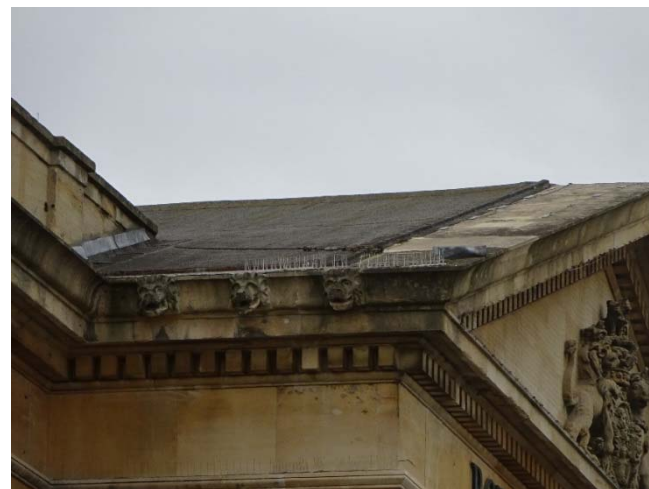
Figure 6: Overlaid bitumen asphalt sheeting to East slope of portico roof.
