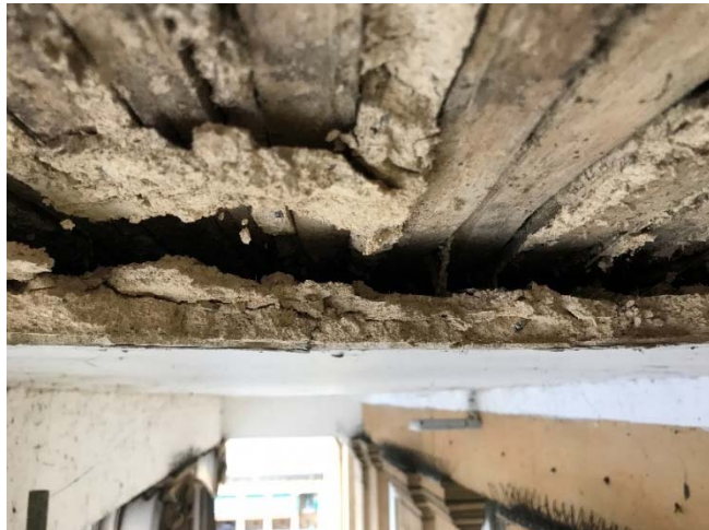
Figure 4: Close-up of edge of missing plaster; showing further loose material at risk of falling away from lath substrate.
