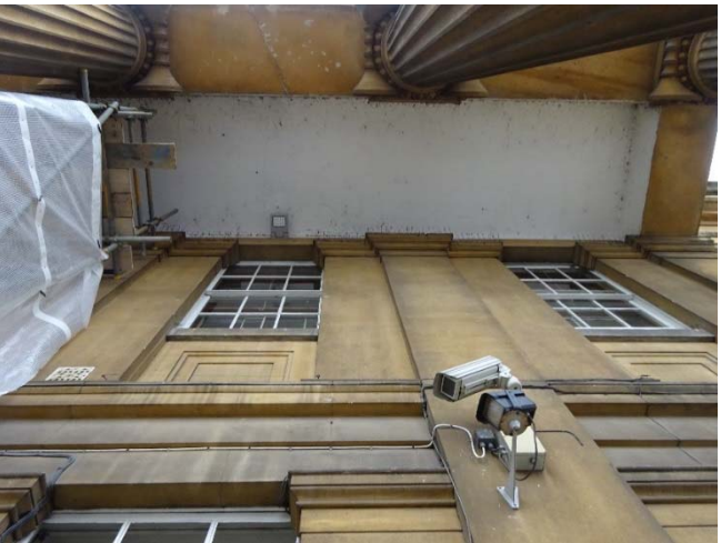
Figure 3: Western end of portico soffit which may also contain areas of loose / live plaster.
