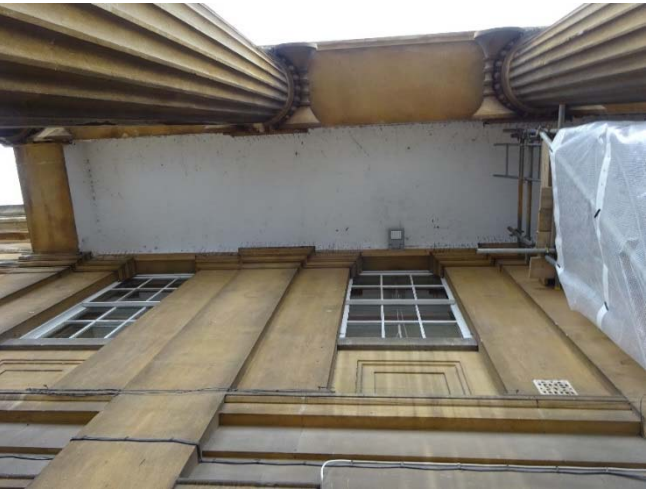
Figure 2: Eastern end of portico soffit which may also contain areas of loose / live plaster.
