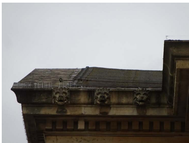
Figure 5: Portico roof viewed from the west showing overlaid possibly deteriorated bitumen asphalt sheeting.
