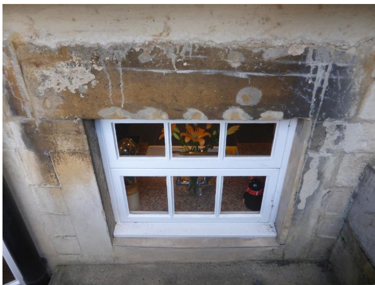
Figure 11: Poor quality repairs to the jamb and lintel of the window and infilling to the lower half
