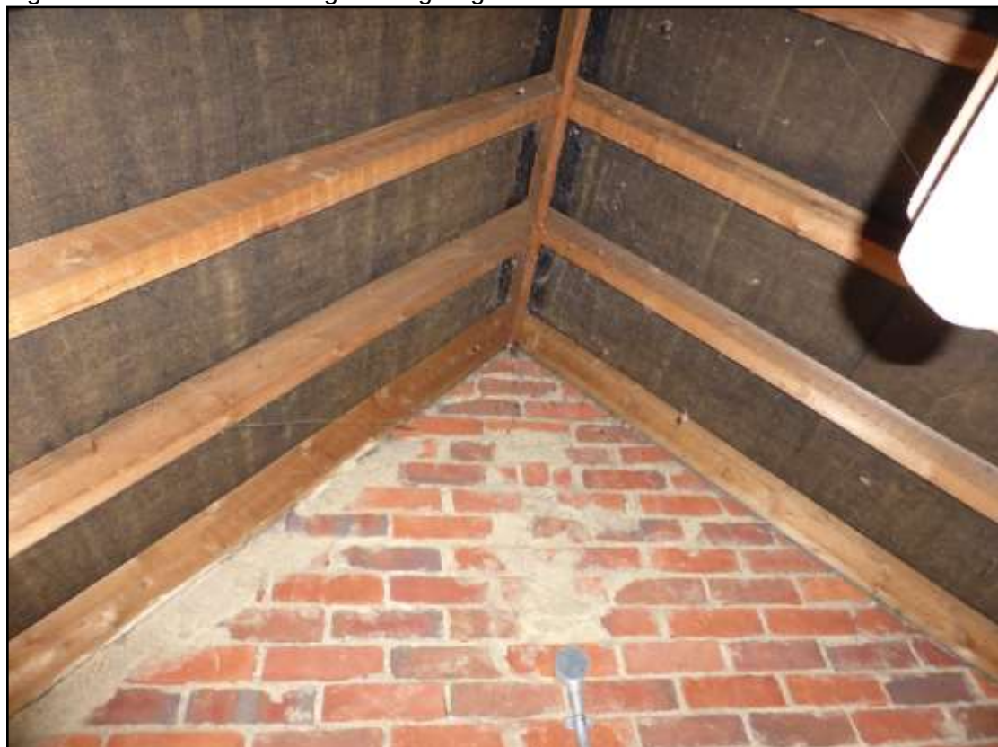
Figure 11. Bitumen felt lining in the garage at 63 Allcroft Road. 21.7.17
