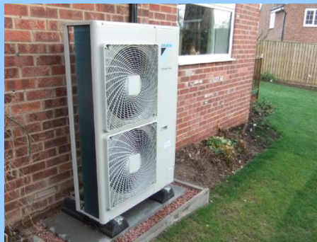
AIR SOURCE HEAT PUMPS
