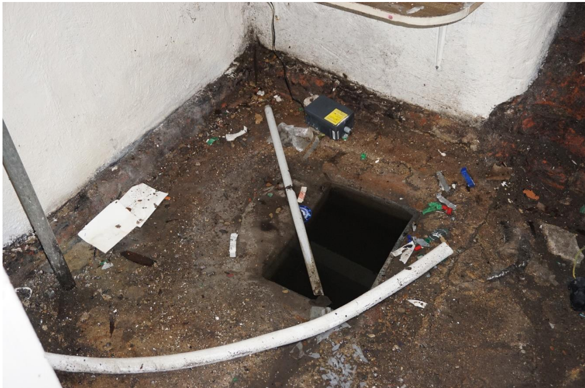
Photograph 17 – Water build up in basement
