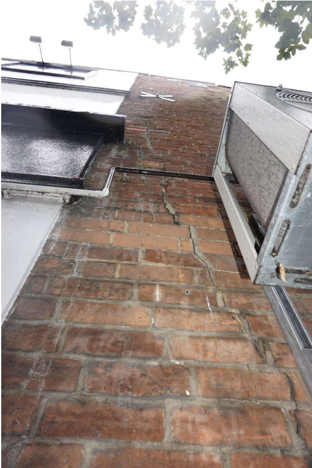
Photograph 6 – Full height crack to gable wall
