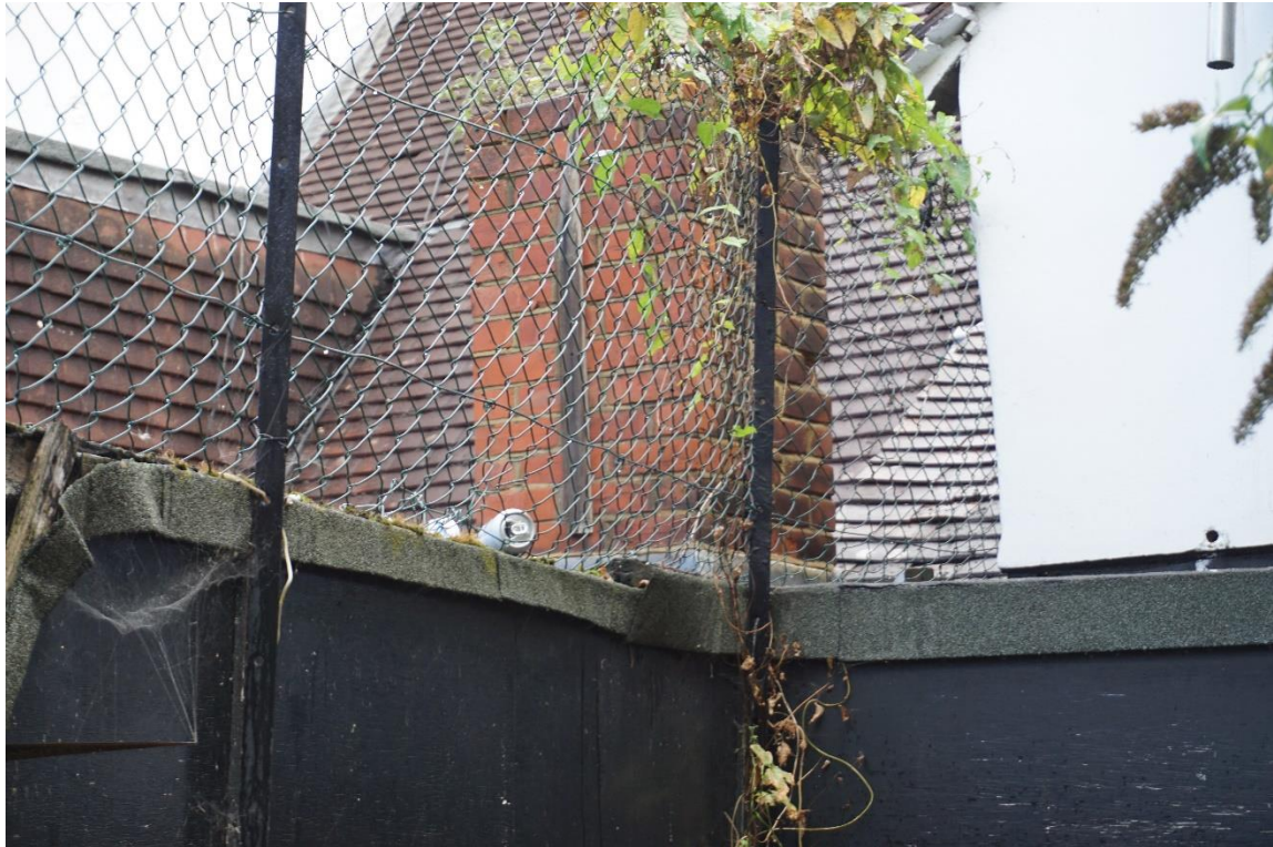
Photograph 11 – Chimney in poor condition
