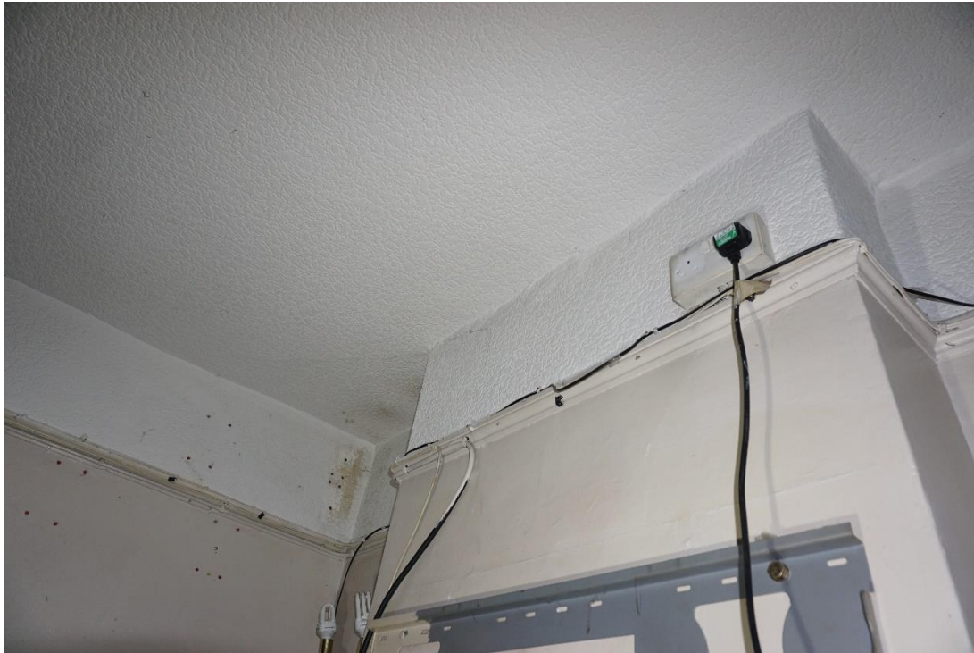
Photograph 18 – Displacement to wall at ceiling junction
