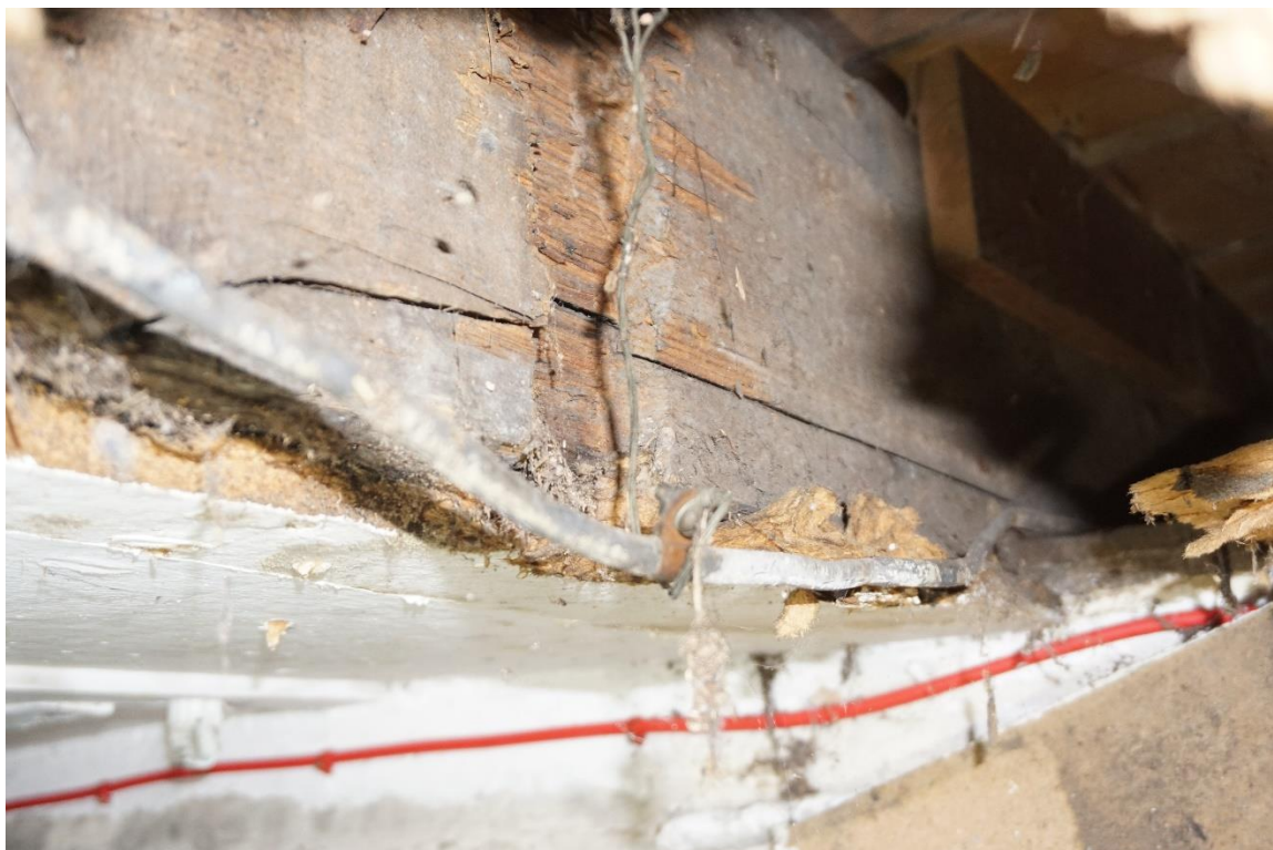
Photograph 12 – Split to floor joist at midspan
