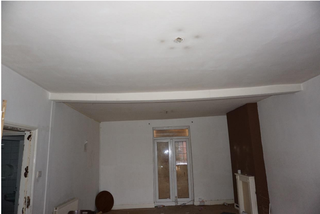
Photograph 20 – Deflection to beam supporting second floor
