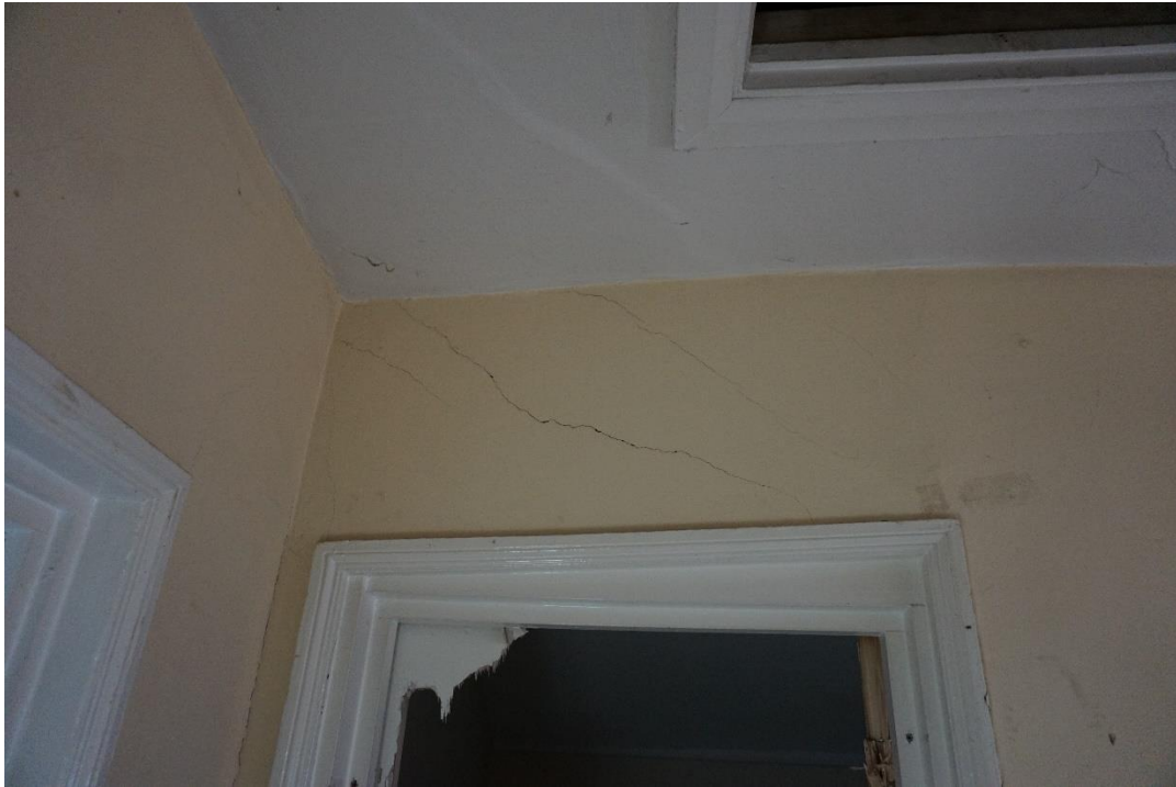
Photograph 22 – Diagonal cracking to wall, note displacement to door frame
