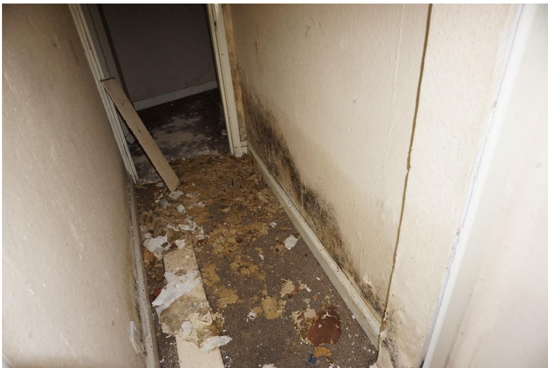
Photograph 19 – Damp to walls
