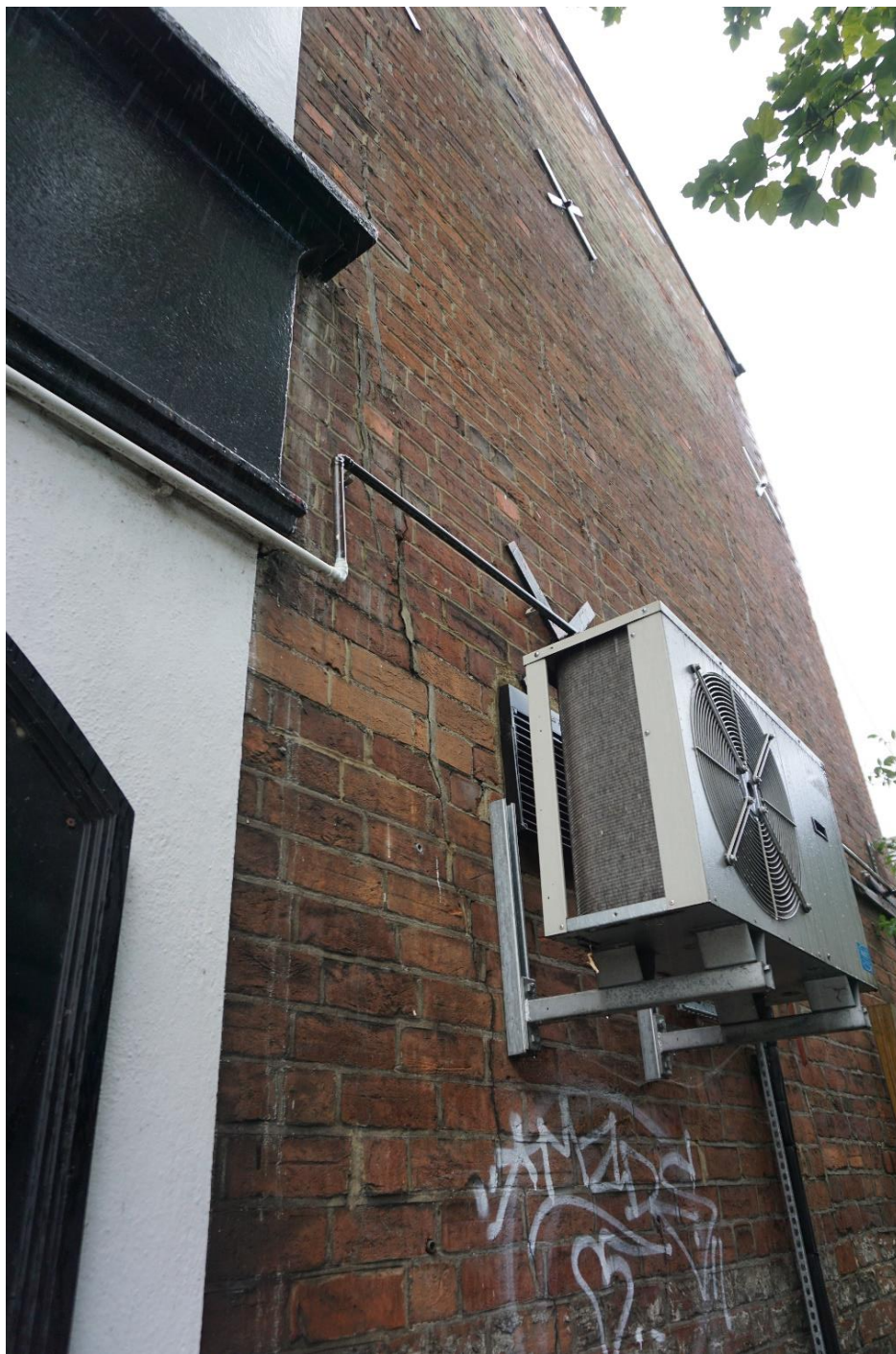
Photograph 7 – Displacement of wall at crack position
