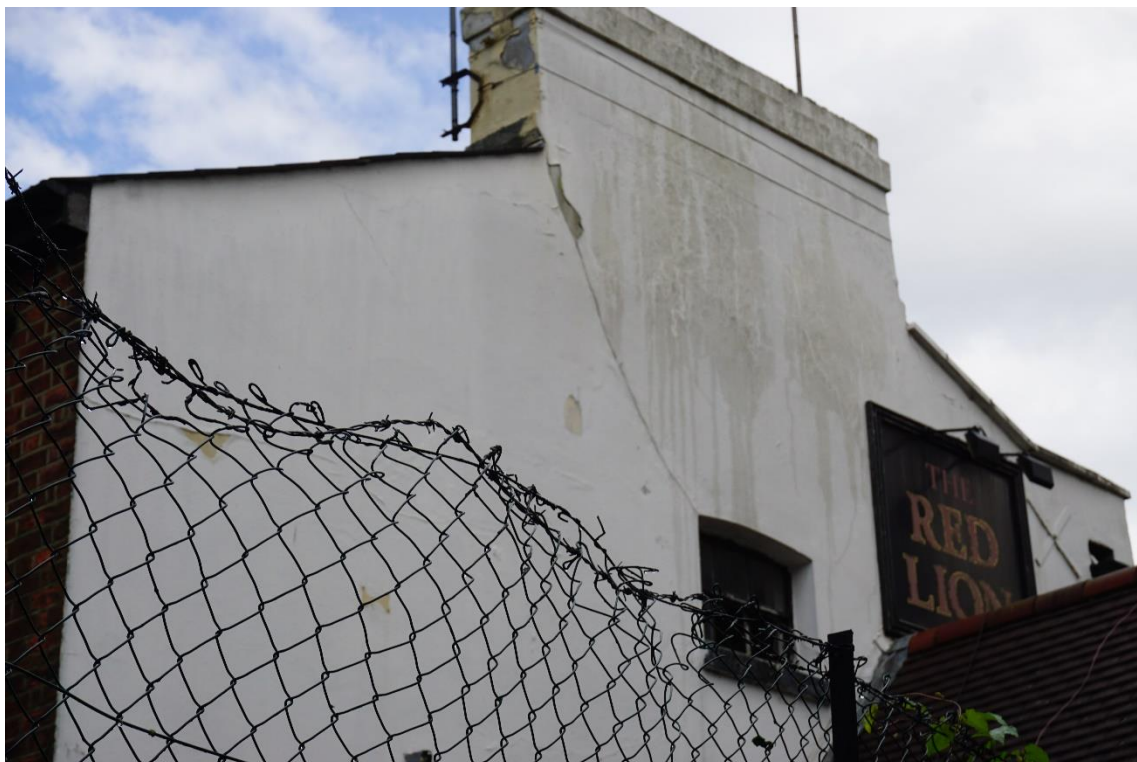
Photograph 9 – Cracking to left hand Gable
