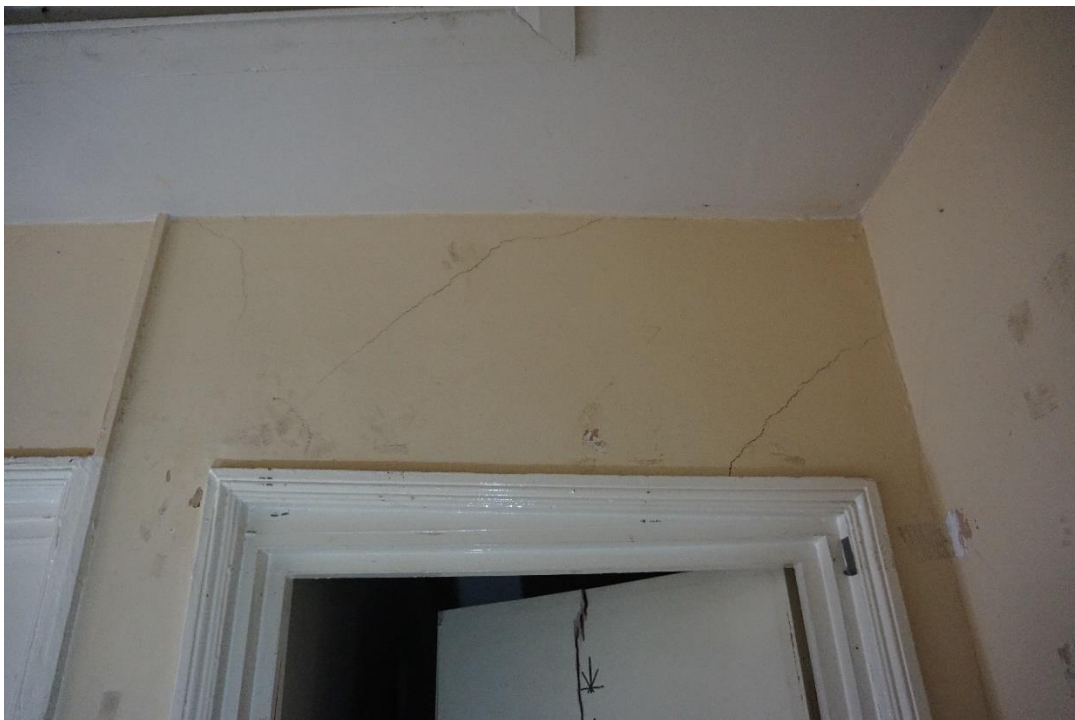
Photograph 23 – Diagonal cracking to wall, note displacement to door frame
