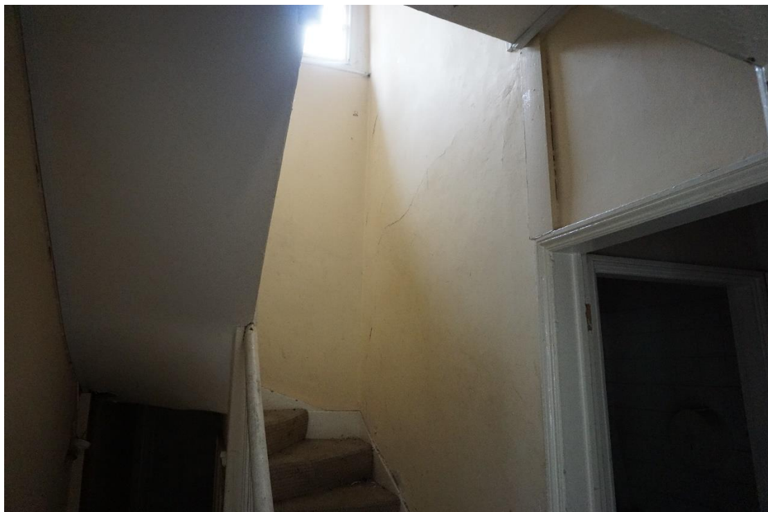
Photograph 21 – Bulging/cracking to stair wall
