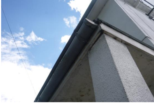
9. Cobwebbed gap at the corner of the porch.
