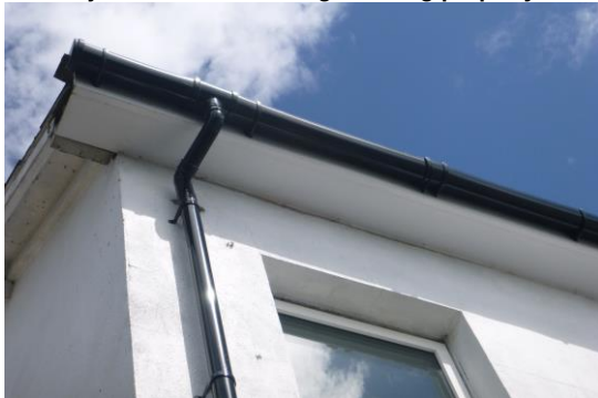
5. The tight UPVC soffit box on the rear of the property.
