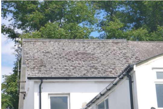
3. Tightly fitted tiles with one slipped tile close to the junction with the neighbouring property.
