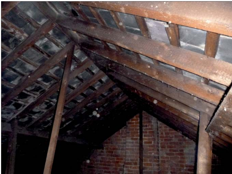
Photograph 4: Showing one of the cobwebbed and unlined roof spaces present (main building at the front of the site).
