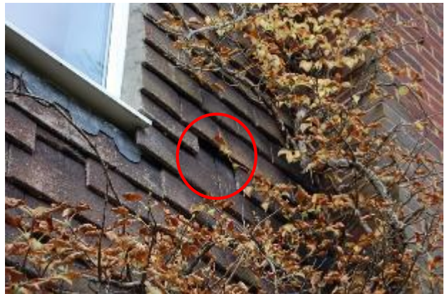
Photograph 4. A crevice feature at the eastern elevation of the dwelling created as a result of a missing hanging tile.
